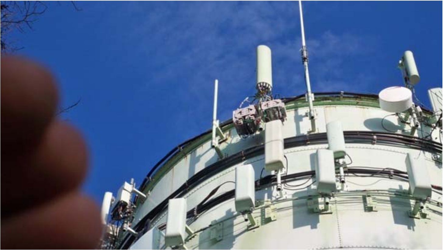
Existing Antenna Installation (uppermost antenna)
