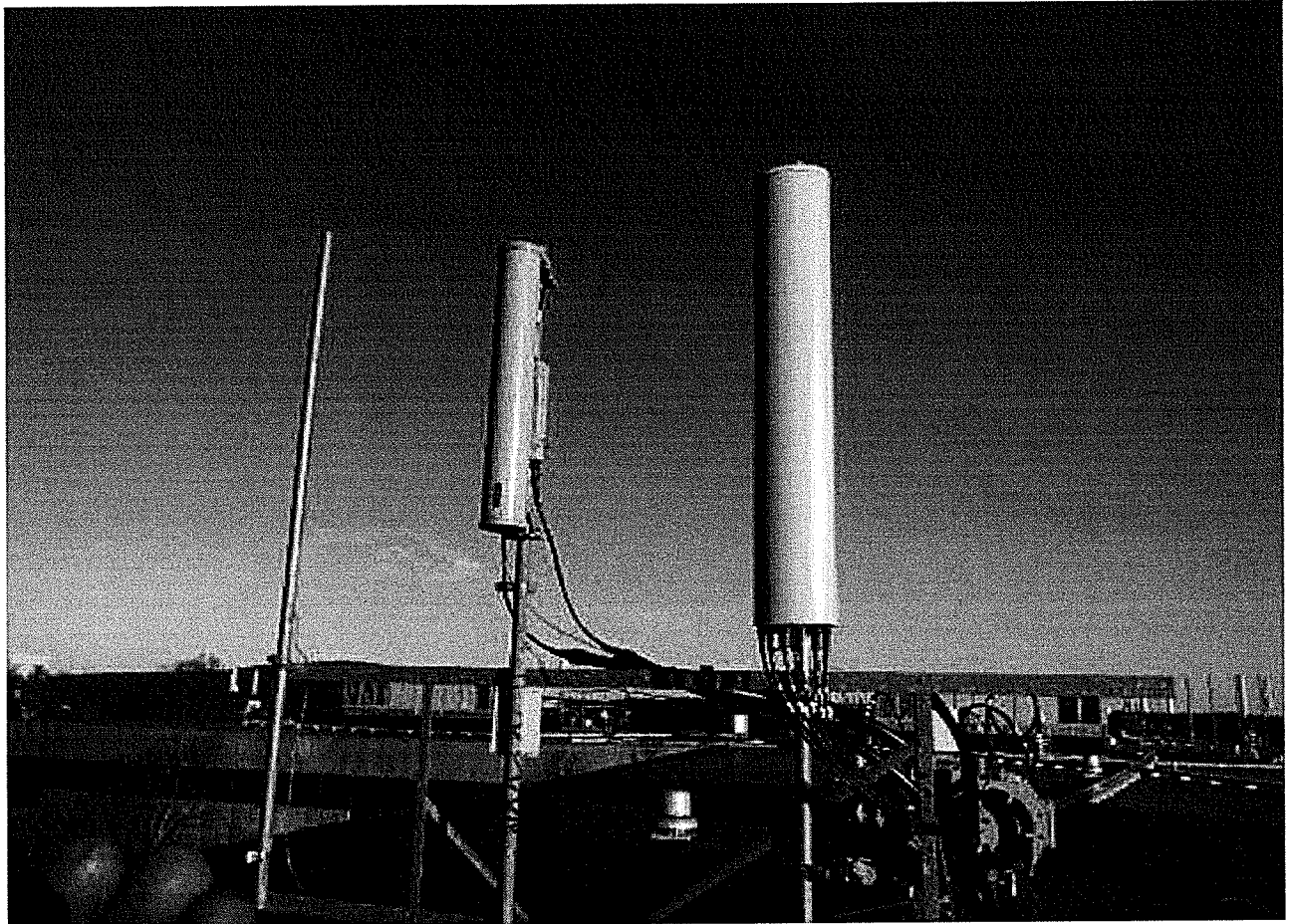
Existing Gamma Sector Antennas
