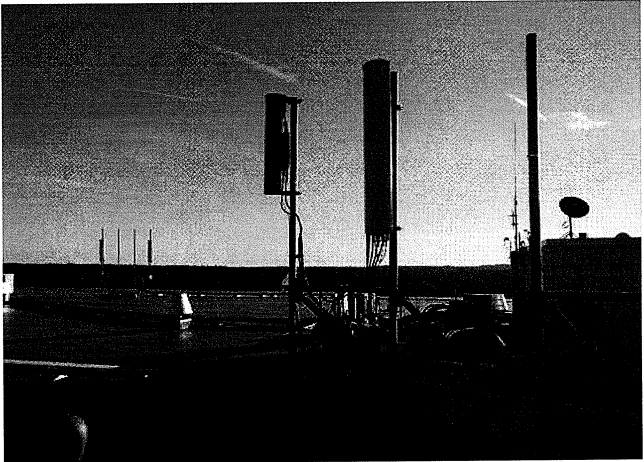
Existing Alpha Sector Antennas
