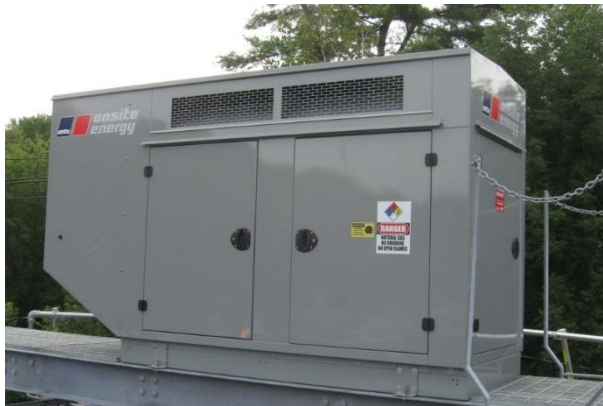
A field image of an MTU 30 kW generator proposed for the East Street site.
