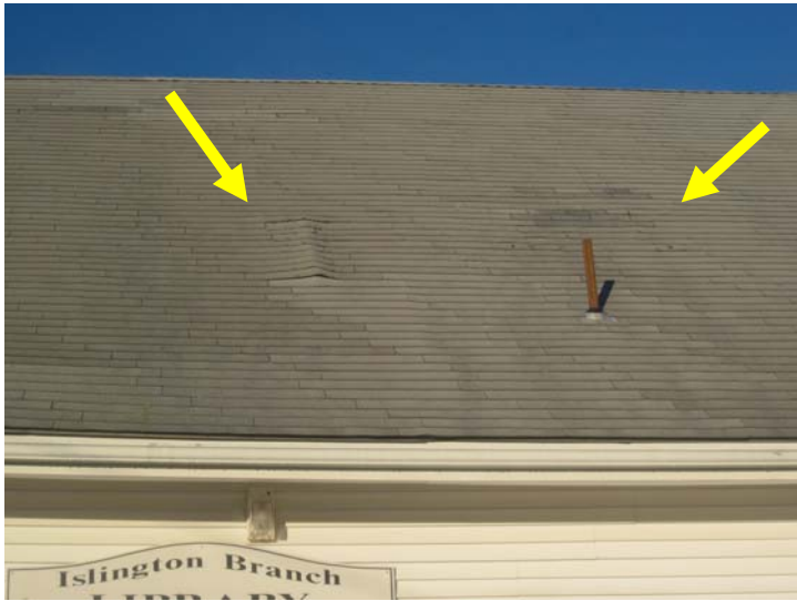
The ageing roof shingles are lifting in several spots providing an access for wind driven rain which has resulted in visible interior moisture damage.
