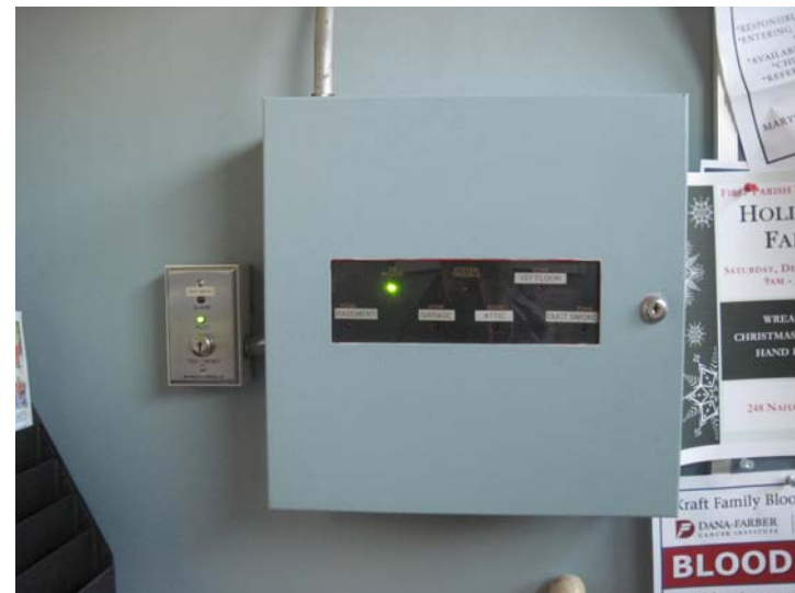
The aging zone-type fire alarm control panel has surpassed its twenty-year expected useful service life and is in need of near-term replacement.
