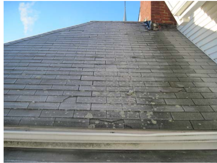
View of significant organic growth and shingle damage at the garage extension roof.
