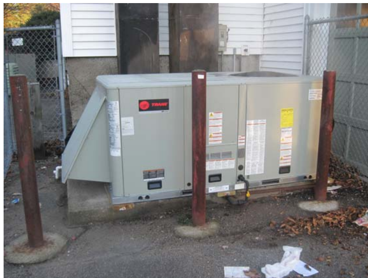
A Trane packaged 130-MBH natural gas heating, 5-ton electric cooling unit was newly installed in 2016 and provides heating and cooling for the entire building.
