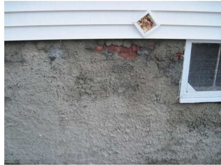
View of the aging, delaminating parging over the original brick foundation at the south end-elevation of the building. In need of near-term removal, as-needed repointing, and complete re-parging.
