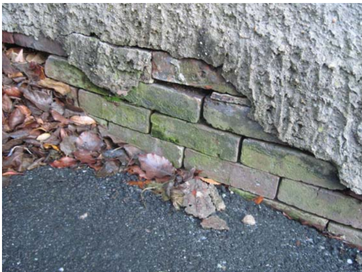
Close-up of complete mortar loss visible at the exposed brick foundation at the south end-elevation. In need of near-term removal, repointing, and re-parging.
