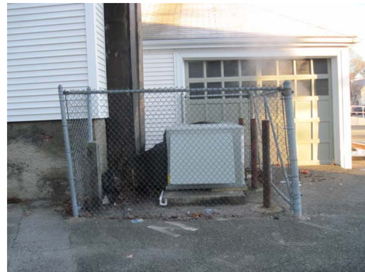
Fencing is limited to the chain link enclosure at the exterior pad-mounted heating/cooling unit. The posts are out of plumb due to vehicle impact and/or snow removal efforts and are in need of repair/re-setting.
