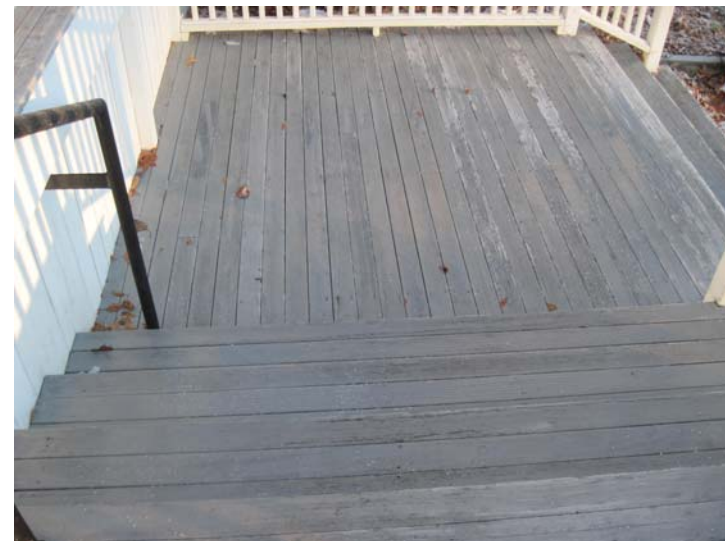
View of aging wood decking boards at the rear-elevation entrance deck structure.
