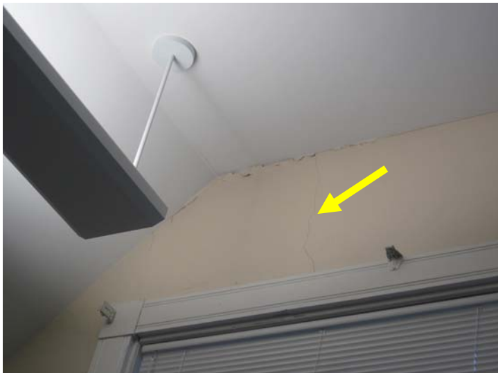
View of wall cracking and paint failure visible at the south-elevation wall.
