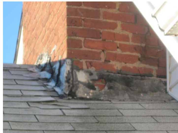
Close-up of deteriorating flashing, cracked bricks, mortar loss, and lifting shingles at the north and east sides of the chimney providing access for wind-driven rain and moisture damage.
