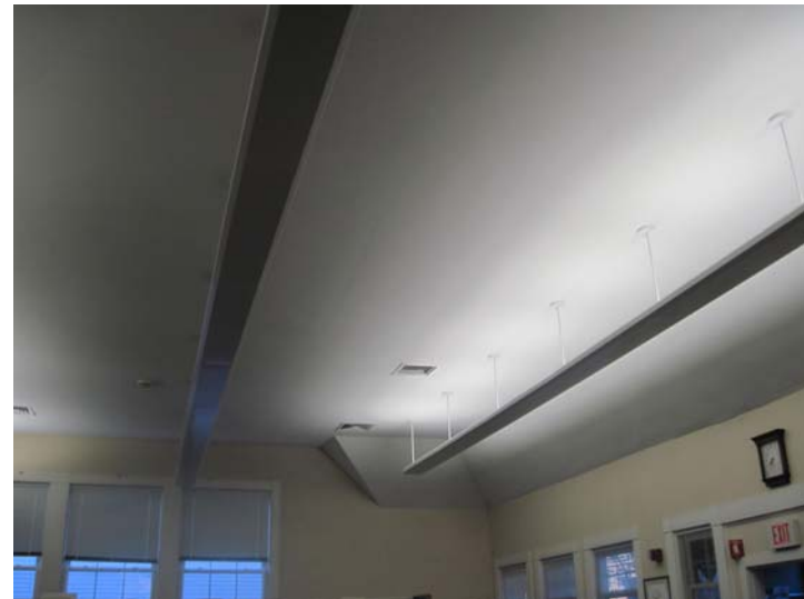
Diffused lighting fixtures were installed during the 1996 renovations.
