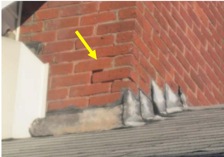
View of visible mortar loss at the chimney's south side.
