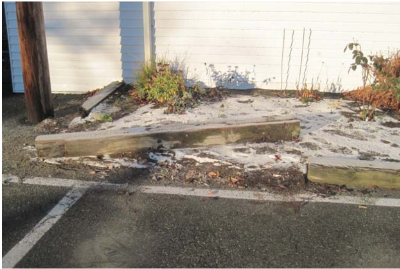
The aging, rotting, damaged rear-elevation landscaping timbers are in need of replacement.
