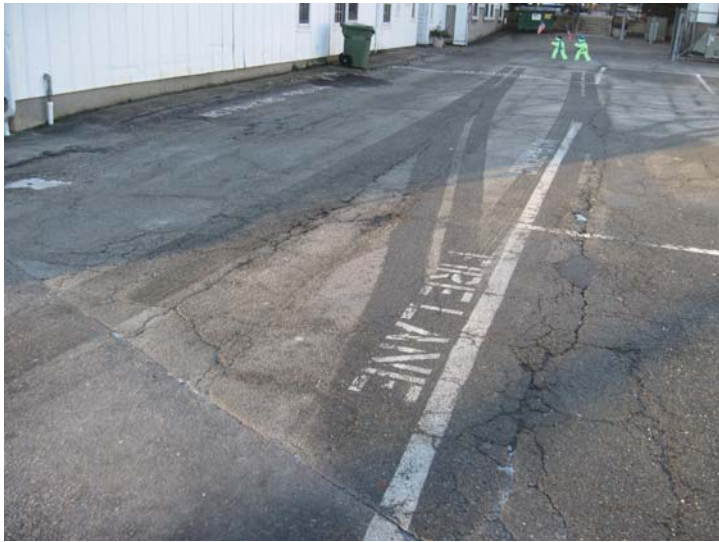
View of the ageing, deteriorating parking lot and fire-lane asphalt surface conditions.
