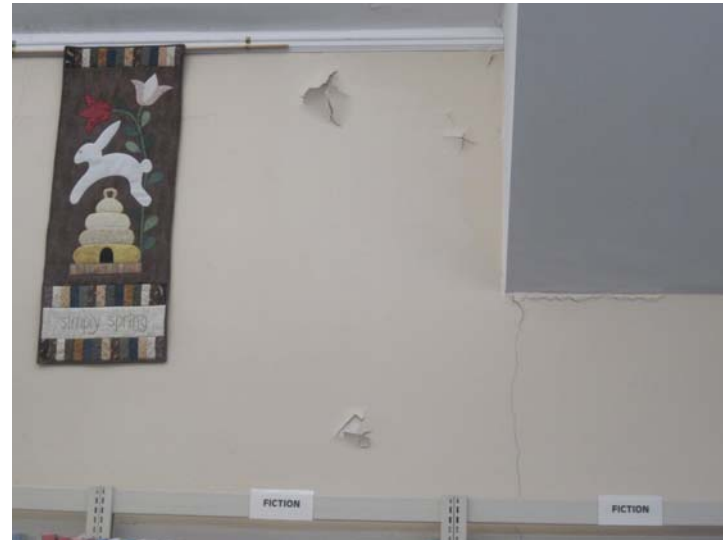
View of moisture-related paint failure and cracking visible along the east-elevation wall.
