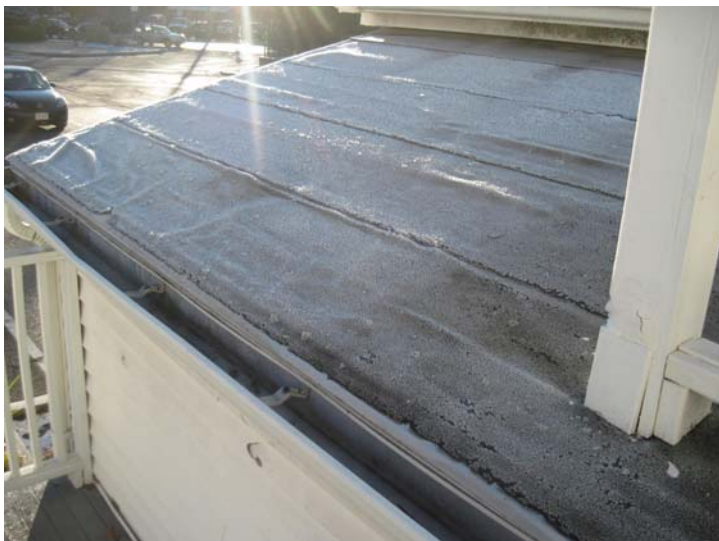
A small section of asphalt roll roofing over the garage structure is also ageing, deteriorating and in need of near-term replacement.
