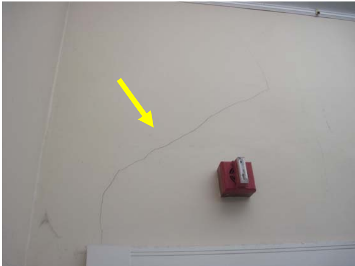
View of cracking wall plaster visible above the rear entrance door.
