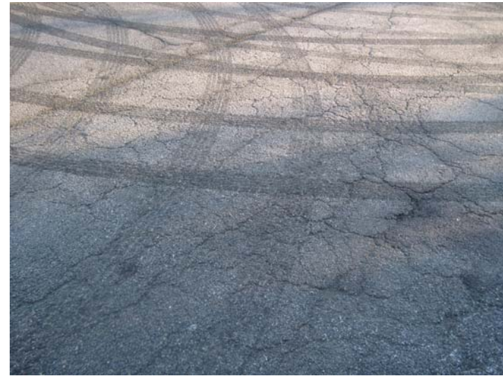
Significant cracking and alligating of the entire asphalt surface is beyond repair. Near term complete resurfacing is recommended.
