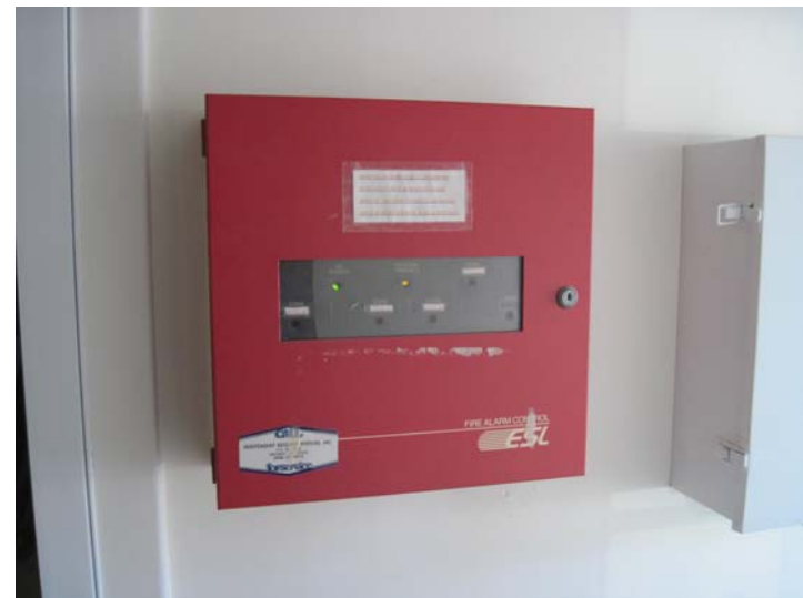
The aging ESL zone-type fire alarm control panel is reportedly greater than twenty years old and in need of near term replacement.
