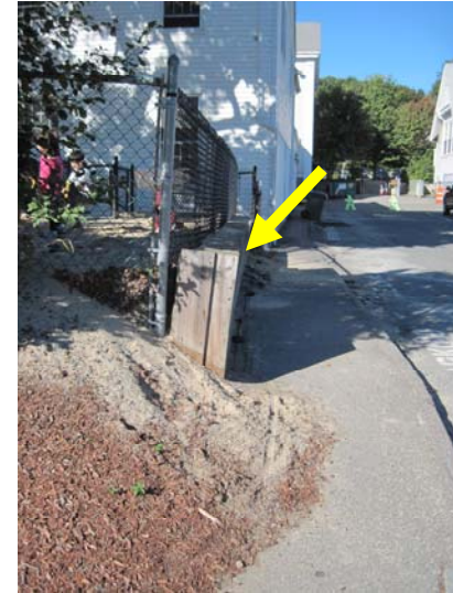
View of the asphalt walkway and adjacent outward leaning timber retaining wall at the east elevation nursery school playground (in need of rebuilding) with mix of older and newer chain link fencing above.
