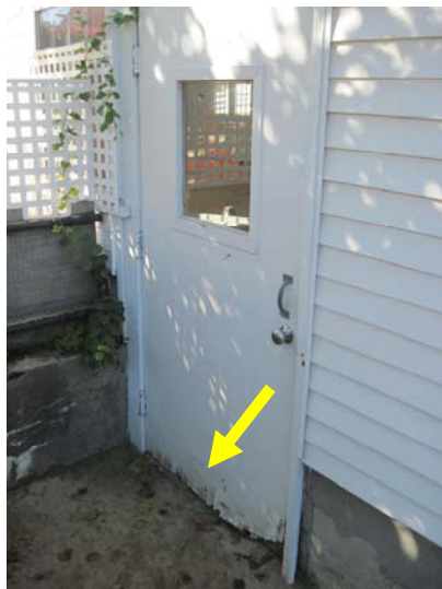
The east elevation egress door from the nursery school auditorium out to the playground exhibits significant base rot and is in need of near term replacement.
