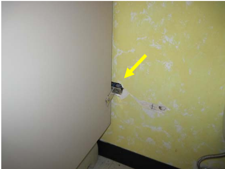
View of damaged partition wall anchor. Both bathrooms are in need of near term renovation.
