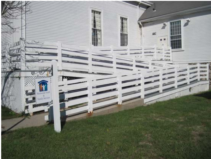
The south elevation accessible ramp exceeds current pitch and rise requirements (1:12 max pitch and 13" max rise) and lacks compliant slip resistance and level resting areas at every 12-feet of run.
