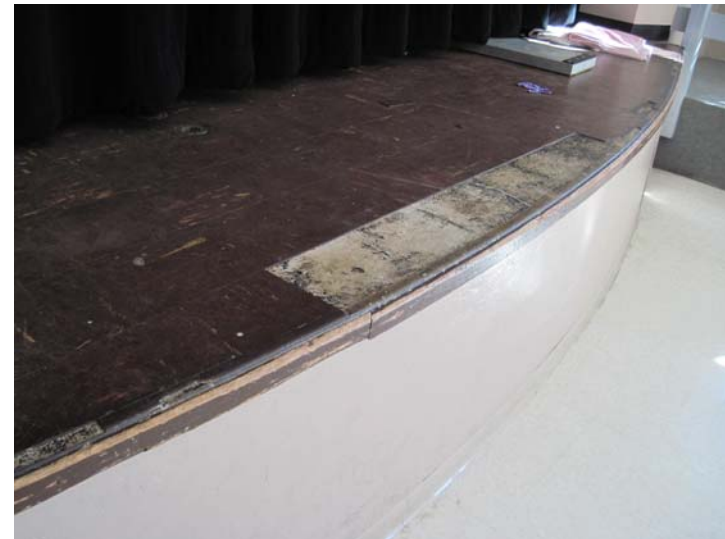
View of the original aging damaged auditorium stage tiles. Tiles are 9"x9" in dimension and could possibly be constructed of asbestos containing material (ACM).
