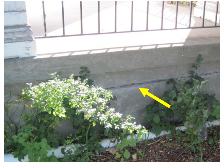
View of exposed cold joint at the sanctuary front entrance porch, in need of near term patching/repair.
