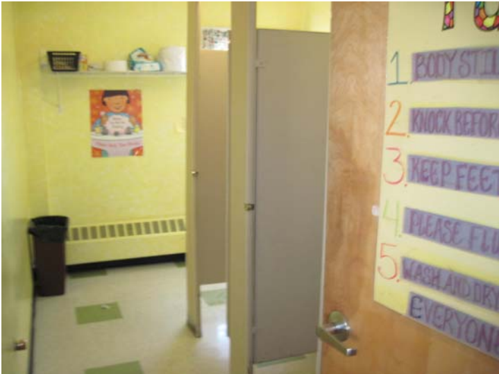
View of ageing nursery school bathroom finishes.
