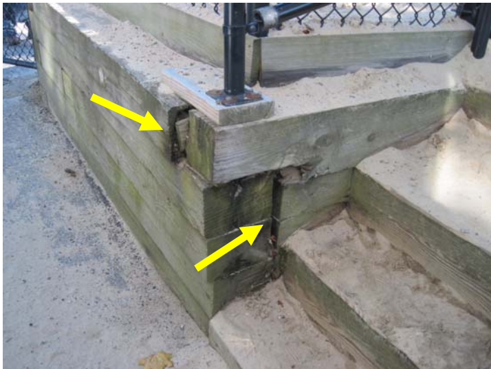
The west facing leg of the timber retaining wall is also damaged with visible outward movement.
