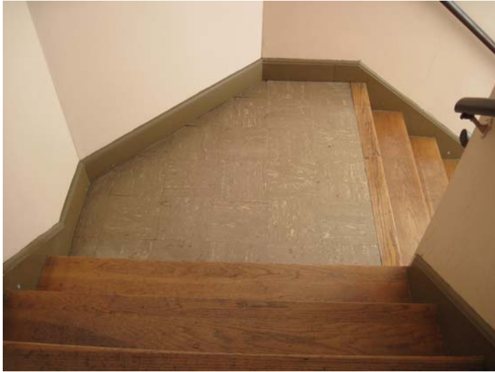
View of the aging wood stair treads and suspected ACM tile landings at the south elevation of the auditorium leading up to the 2 nd Floor classrooms.
