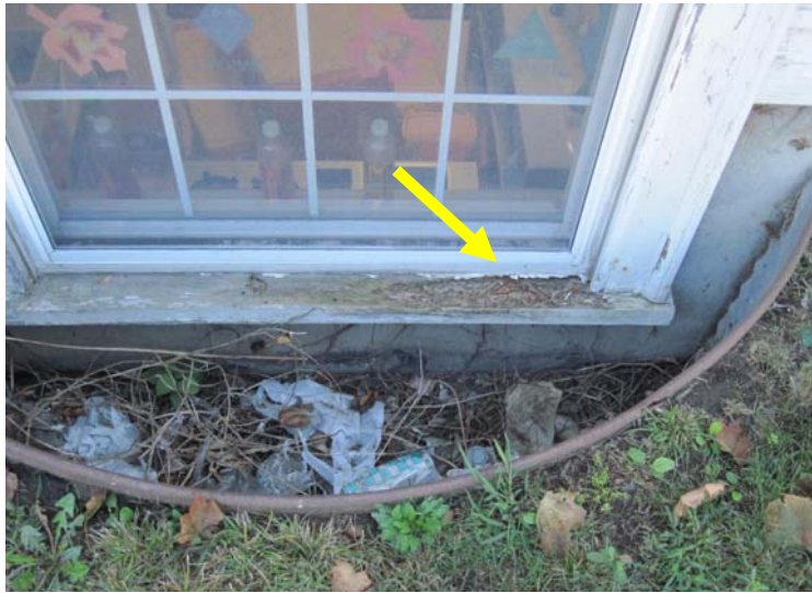
Rotting wood window sills at the sub-grade basement-level windows along the west elevation are all in need of near term replacement
