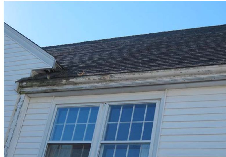
View of rotting wood gutters and aging 3-tab asphalt shingle roofing at the north elevation.
