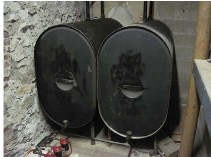
The boiler fuel oil is stored in two 330-gallon above-ground residential oil tanks. Both are estimated to be greater than 20-years old.
