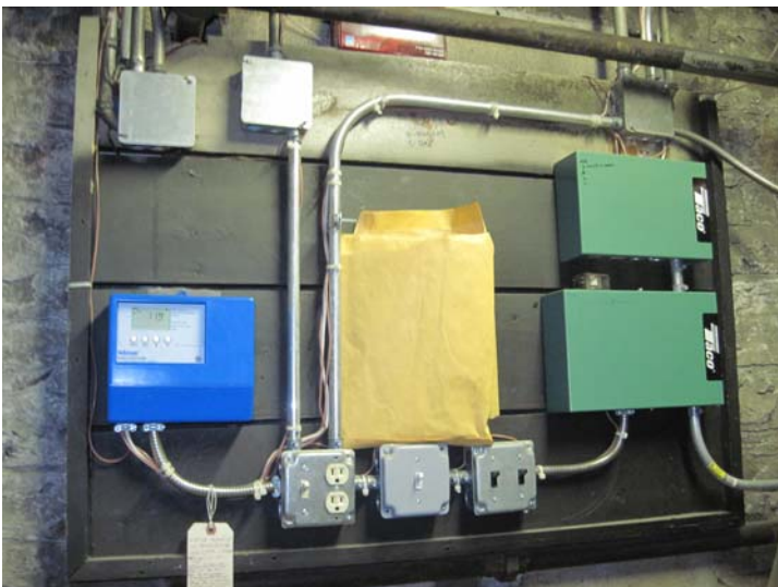
Controls include a Tekmar 264 modulating boiler control panel (blue, left) and Taco SR504 and SR506 zone switching relay panels (green, right).
