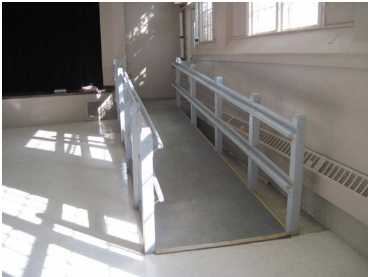
The aging accessible ramp does not meet current requirements and is in need of near term replacement.
