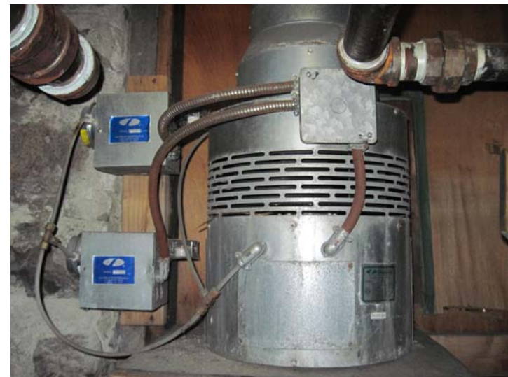
A Field Controls CAS-6 thermostatically controlled "Fan-in-a-Drum" combustion air system automatically draws combustion air into the boiler room when needed and sends a signal to the burners when ok to fire.
