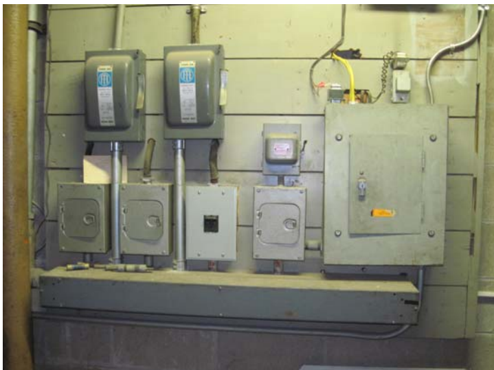
View of the building electrical distribution equipment and disconnect switches.
