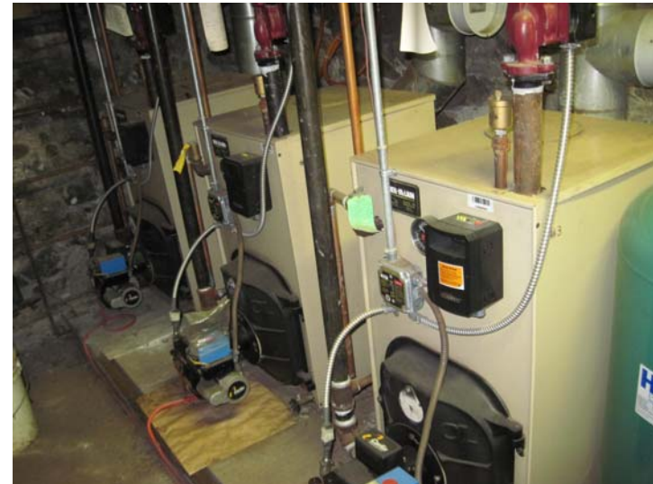
Building heat is provided by a trio of Weil-McLain Gold WGO-6, 212-MBH oil-fired hot water boilers with a series of fractional horsepower in-line boiler and heating water cartridge circulators.
