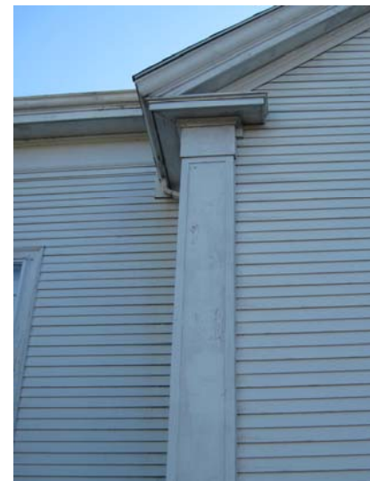
Close-up of aging trim paint in need of surface near term preparation and painting and aging, dirt-covered, clapboard profile vinyl siding.
