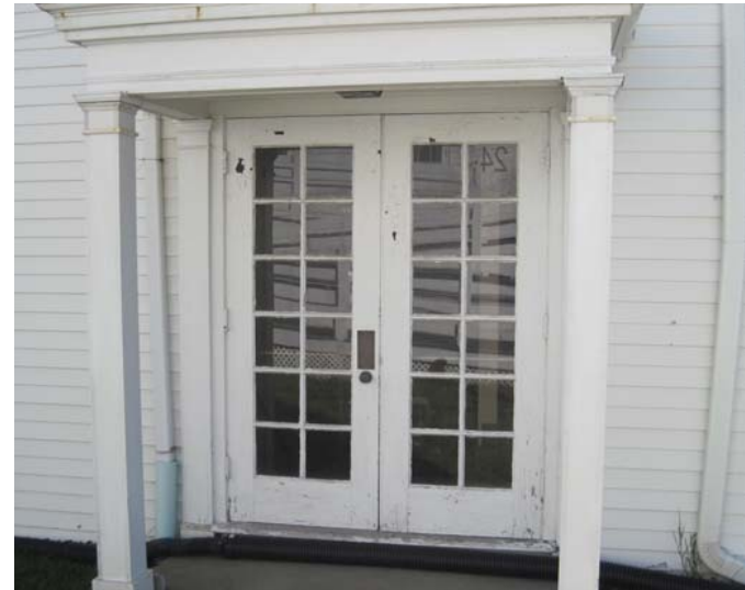
The aging double leaf wood French doors at the 1960's addition west elevation entrance are in need of near term replacement.
