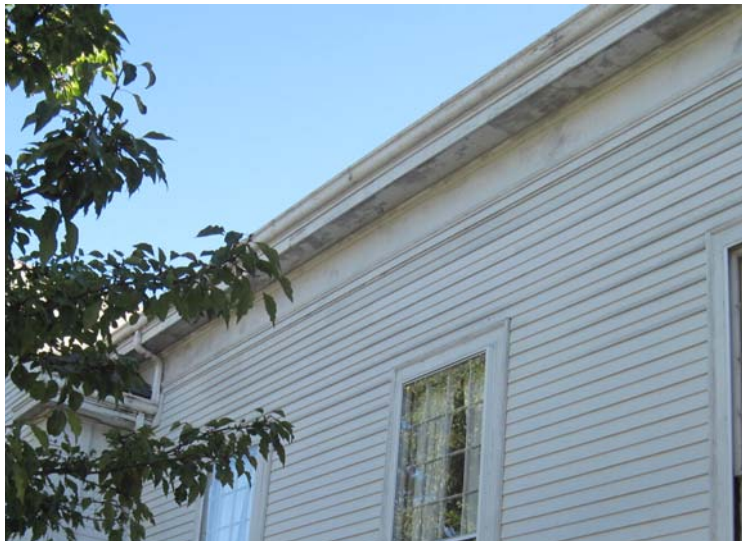
View of failing soffit paint and aging, damaged original wood gutters, in need of near term replacement.
