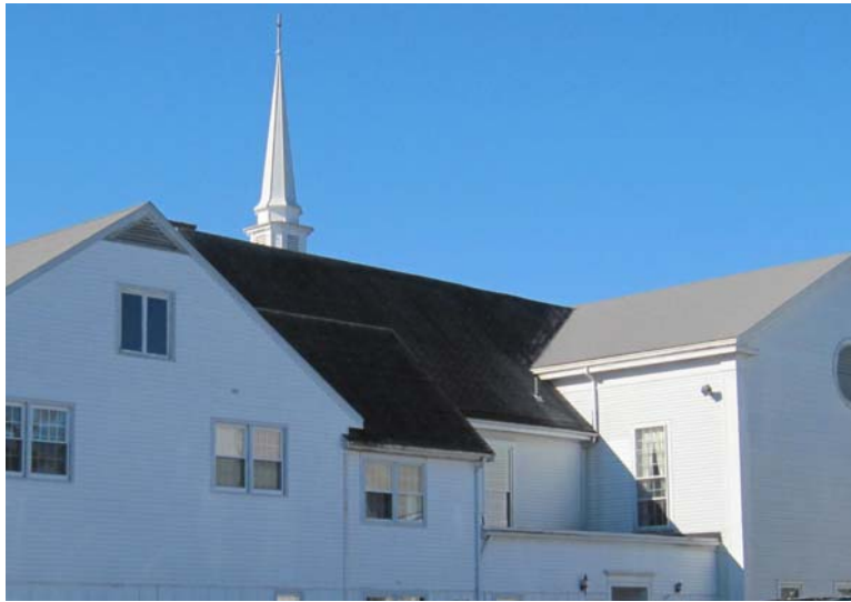
The 3-tab asphalt shingle roofing exhibits mixed conditions with the most severe aging visible along the north elevation over the main entrance.
