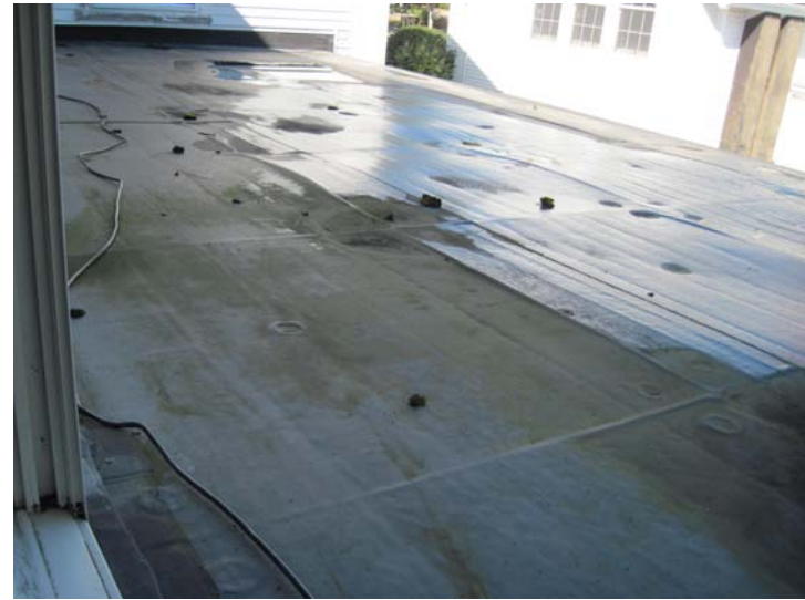
View of the aging mechanically fastened EPDM rubber membrane over the main entrance flat roof structure.
