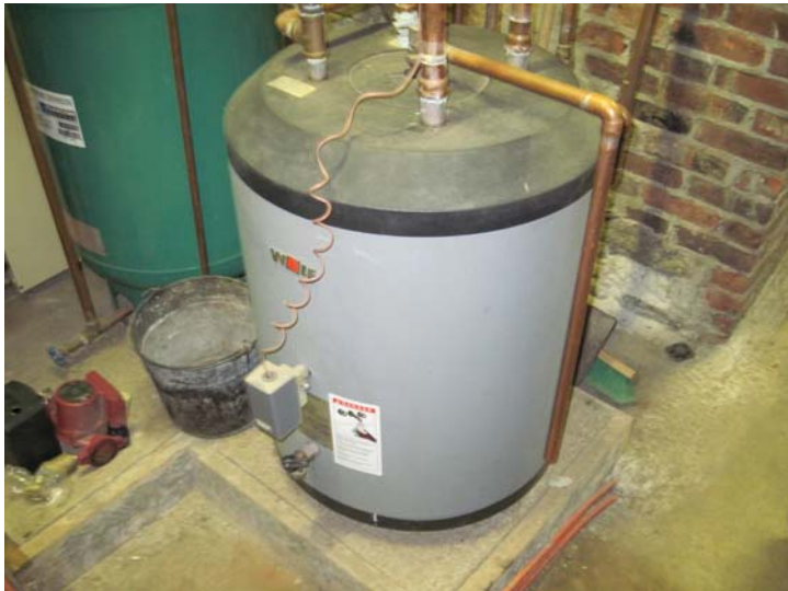
Domestic hot water is produced by a Wolf 30-gallon lowboy indirect-fired hot water storage tank with internal water to water heat exchanger.
