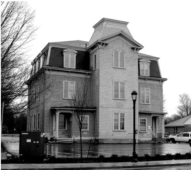
The Colburn School with new Mansard roof and Plexiglas window protection completed.
