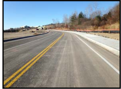
The “new” Rosemont Rd. west of University Avenue, slated to open (weather permitting) in late January or early February 2014.
