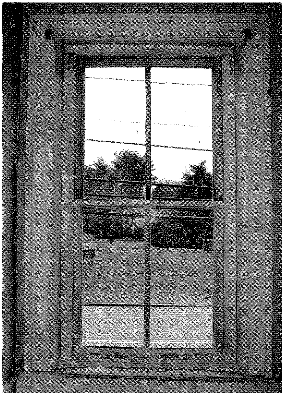
Window view from Obed & Betsey Baker House looking onto Veteran's Park at Pond Street.
