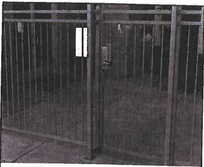
FIGURE 305.2.6(2) VIOLATION—BARRIER (FENCE) HORIZONTAL MEMBERS TOO CLOSE
