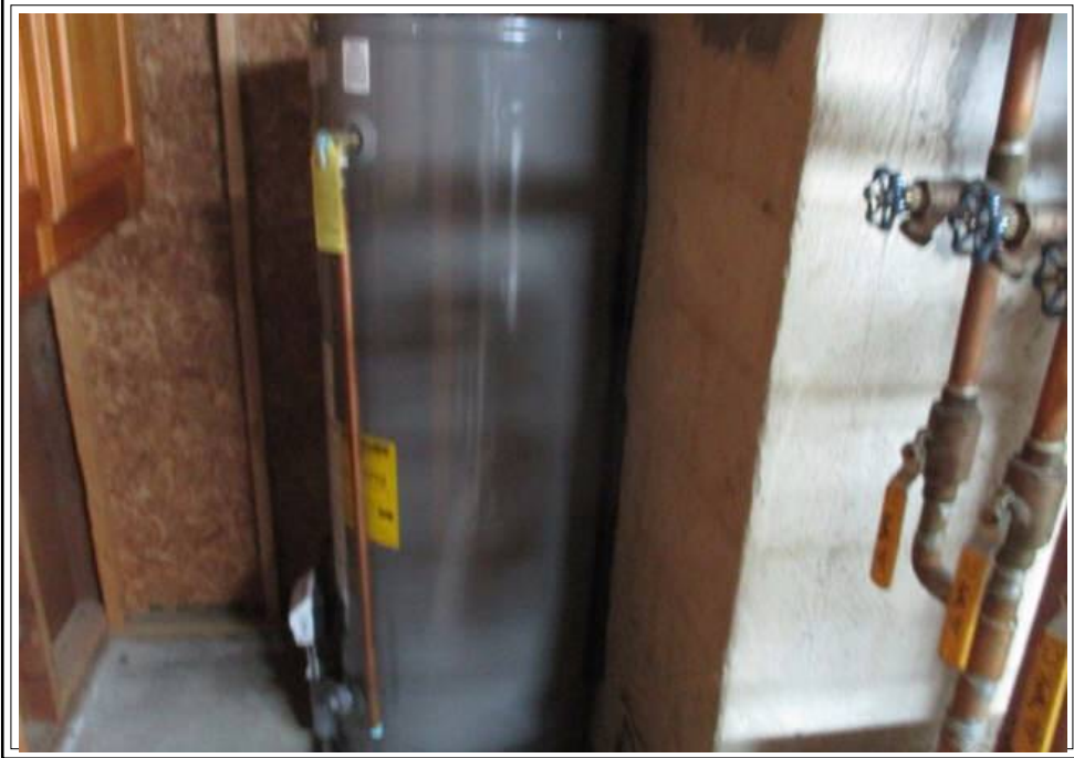
HOT WATER TANK
