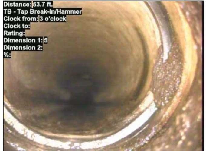
Photo: 15_015-15_016-20230724-135350.JPG At: 53.7 ft. 3/. TB - Tap Break-in/Hammer Joint: No
