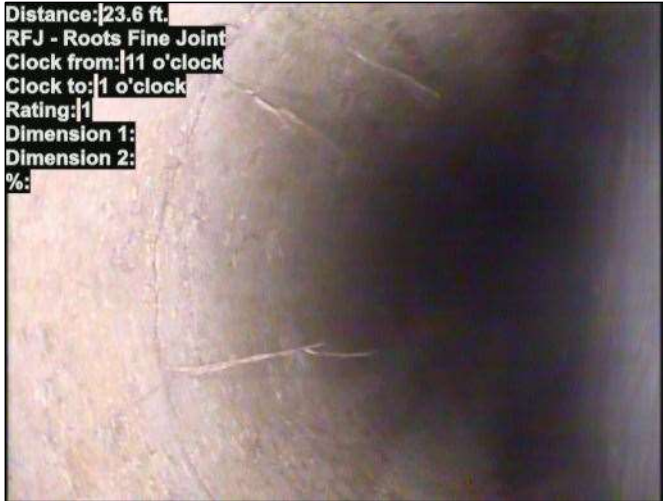
Photo: 15_062-15_081-20230804-124046.JPG At: 23.6 ft. 11/1 RFJ - Roots Fine Joint Joint: Yes
