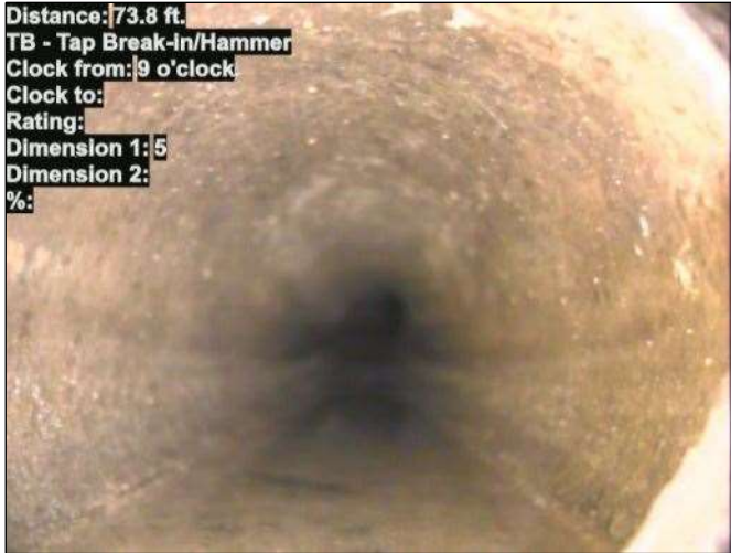
Photo: 15_001-15_002-20230725-121926.JPG At: 73.8 ft. 9/. TB - Tap Break-in/Hammer Joint: No
