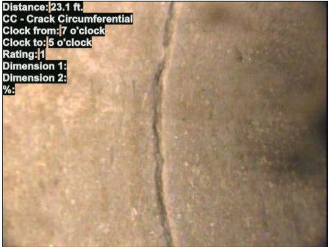
Photo: 15_078-15_061-20230801-082048.JPG At: 23.1 ft. 7/5 CC - Crack Circumferential Joint: No
