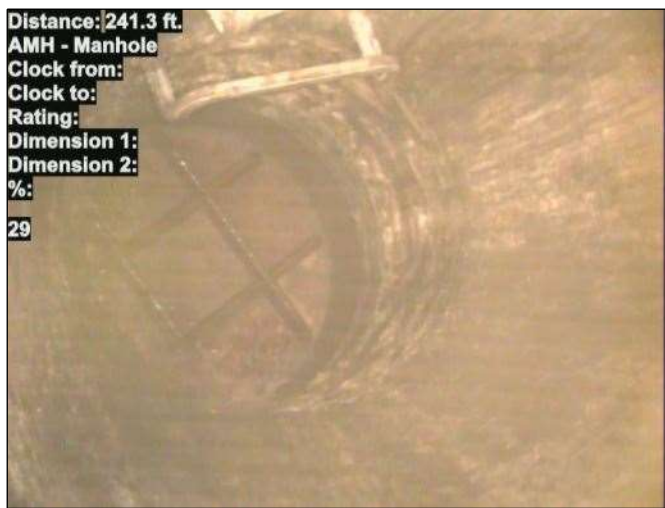
Distance: 241.3 ft. AMH - Manhole Clock from: Clock to: Rating: Dimension 1: Dimension 2: %: 29 Photo: 15_028-15_029-20230724-163834.JPG At: 241.3 ft. AMH - Manhole Joint: No 29
