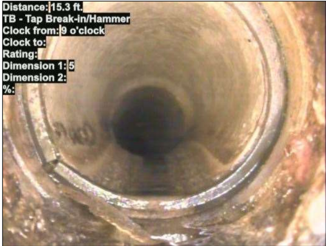
Photo: 15_009A-15_006-20230726-104433.JPG At: 15.3 ft. 9/. TB - Tap Break-in/Hammer Joint: No
