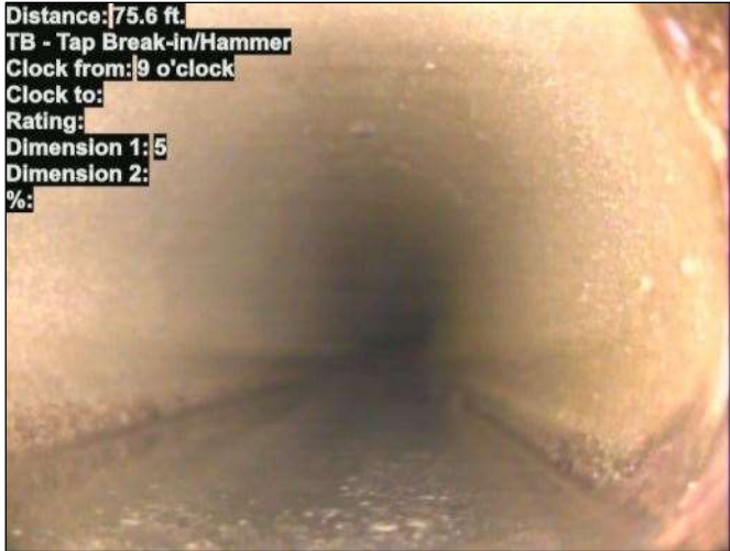
Photo: 15_042-15_043-20230801-130357.JPG At: 75.6 ft. 9/. TB - Tap Break-in/Hammer Joint: No
