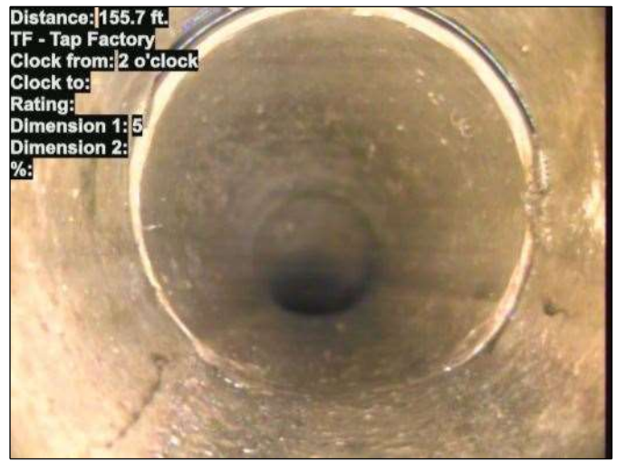
Distance: 155.7 ft. TF - Tap Factory Clock from: 2 o'clock Clock to: Rating: Dimension 1: 5 Dimension 2: %: Photo: 15_016-15_017-20230724-140839.JPG At: 155.7 ft. 2/. TF - Tap Factory Joint: No
