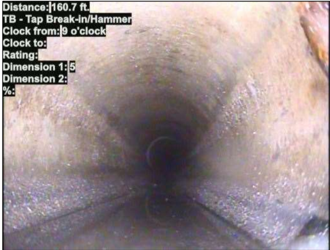
Photo: 15_058-15_059-20230804-073503.JPG At: 160.7 ft. 9/. TB - Tap Break-in/Hammer Joint: No
