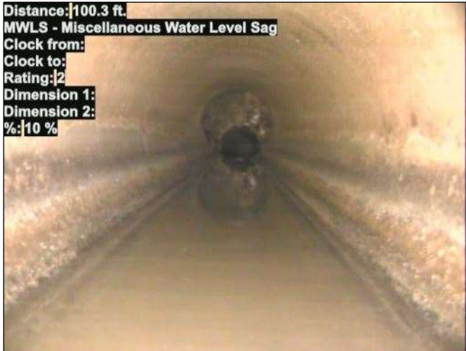
Photo: 15_071-15_072-20230726-082427.JPG At: 100.3 ft. MWLS - Miscellaneous Water Level Sag Joint: No 10 %
