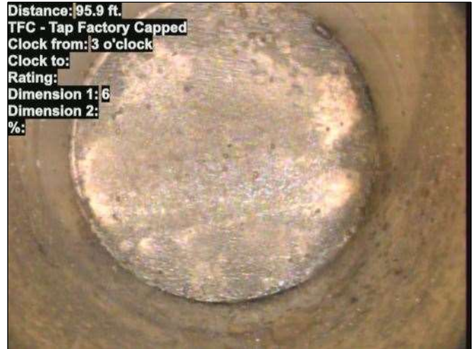
Photo: 15_016-15_017-20230724-140628.JPG At: 95.9 ft. 3/. TFC - Tap Factory Capped Joint: No
