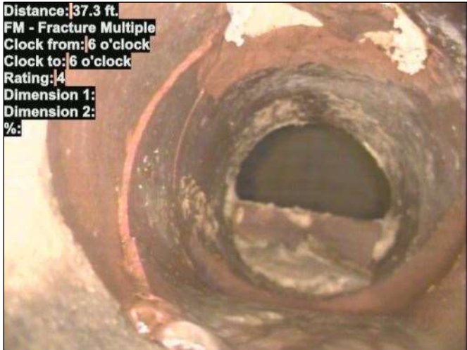
Photo: 15_039-15_040-20230724-124520.JPG At: 37.3 ft. 6/6 FM - Fracture Multiple Joint: No
