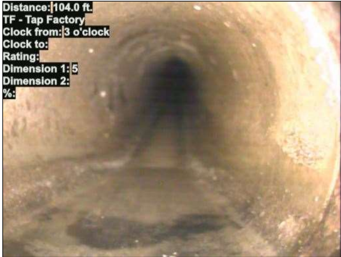
Photo: 15_070-15_071-20230726-081322.JPG At: 104 ft. 3/. TB - Tap Break-in/Hammer Joint: No
