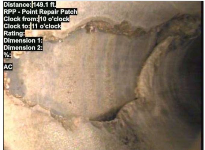
Photo: 15_074-15_075-20230726-084741.JPG At: 149.1 ft. RPP - Point Repair Patch 10/11 Joint: No AC
