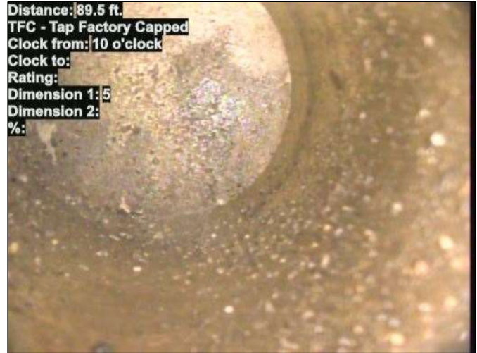
Photo: 15_024-15_033-20230801-101217.JPG At: 89.5 ft. 10/. TFC - Tap Factory Capped Joint: No
