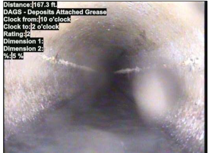
Photo: 15_059-15_060-20230804-085713.JPG At: 167.3 ft. DAGS - Deposits Attached Grease 10/2 Joint: No 5 %
