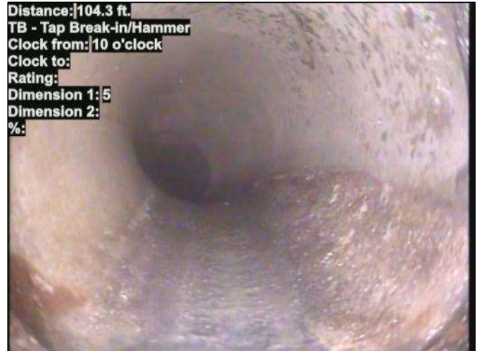
Photo: 15_062-15_081-20230804-122905_1.JPG At: 104.3 ft. 10/. TB - Tap Break-in/Hammer Joint: No
