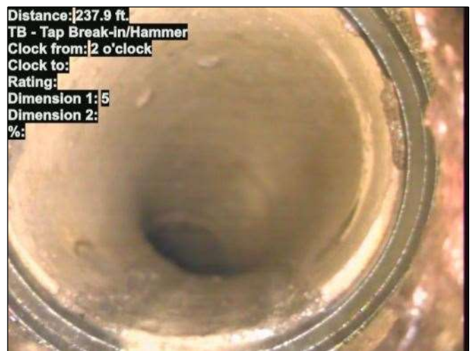
Distance: 237.9 ft. TB - Tap Break-in/Hammer Clock from: 2 o'clock Clock to: Rating: Dimension 1: 5 Dimension 2: %: Photo: 15_014-15_015-20230724-144538.JPG At: 237.9 ft. 2/. TB - Tap Break-in/Hammer Joint: No
