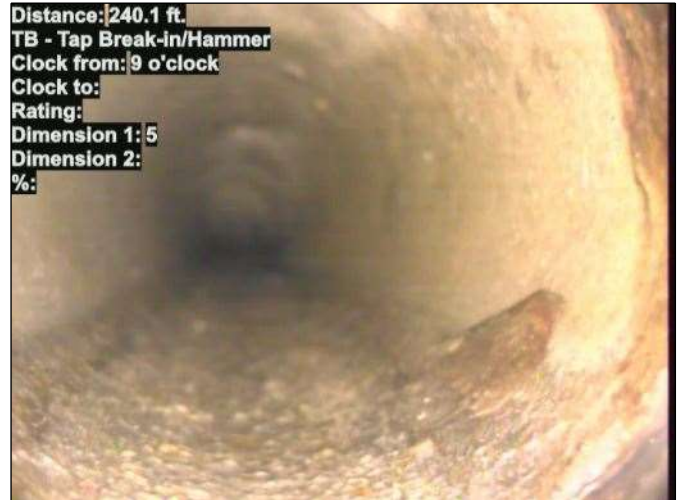
Photo: 15_033-15_034-20230801-105044.JPG At: 240.1 ft. 9/. TB - Tap Break-in/Hammer Joint: No
