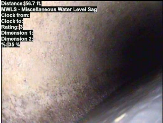
Distance: 56.7 ft. MWLS - Miscellaneous Water Level Sag Clock from: Clock to: Rating: 3 Dimension 1: Dimension 2: %: 35 % Photo: 15_092-15_062-20230804-111229.JPG At: 56.7 ft. MWLS - Miscellaneous Water Level Sag Joint: No 35 %
