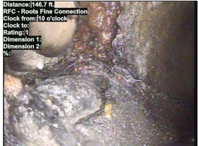
Distance: 146.7 ft. RFC - Roots Fine Connection Clock from: 10 o'clock Clock to: Rating: 1 Dimension 1: Dimension 2: %: Photo: 15_092-15_062-20230804-112815.JPG At: 146.7 ft. 10/. RFC - Roots Fine Connection Joint: No
