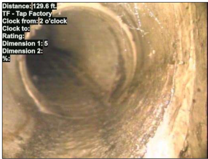
Distance: 129.6 ft. TF - Tap Factory Clock from: 2 o'clock Clock to: Rating: 5 Dimension 1: 5 Dimension 2: %: Photo: 15_019-15_018-20230721-114702.JPG At: 129.6 ft. 2/. TF - Tap Factory Joint: No
