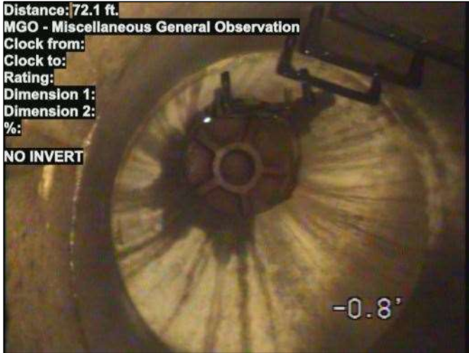
Photo: 15_111-15_112-20230807-102844.JPG At: 71 ft. MGO - Miscellaneous General Observation Joint: No NO INVERT
