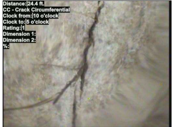
Photo: 15_062-15_081-20230804-121254_1.JPG At: 24.4 ft. 10/5 CC - Crack Circumferential Joint: No
