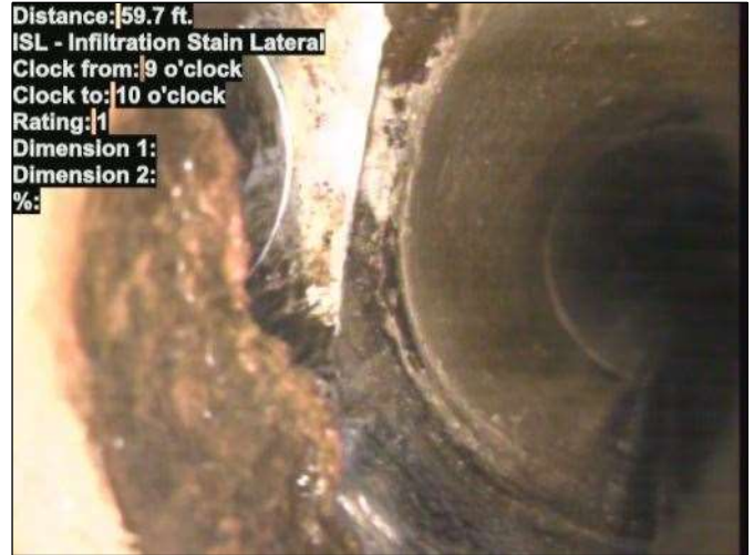
Photo: 15_017-15_018-20230724-150624.JPG At: 59.7 ft. 9/10 ISL - Infiltration Stain Lateral Joint: No
