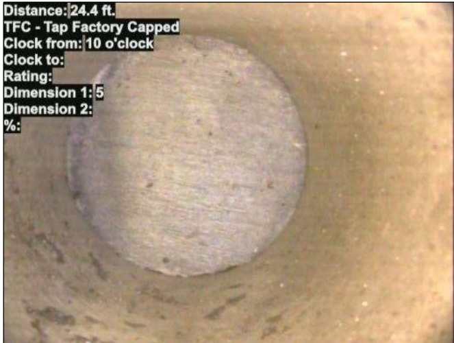
Photo: 15_056-15_057-20230725-074427.JPG At: 24.4 ft. 10/. TFC - Tap Factory Capped Joint: No
