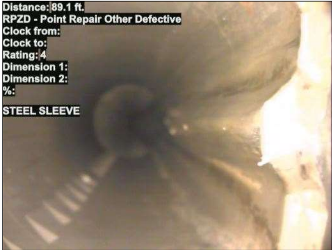
Photo: 15_071-15_072-20230726-082330_1.JPG At: 89.1 ft. RPZD - Point Repair Other Defective Joint: No STEEL SLEEVE
