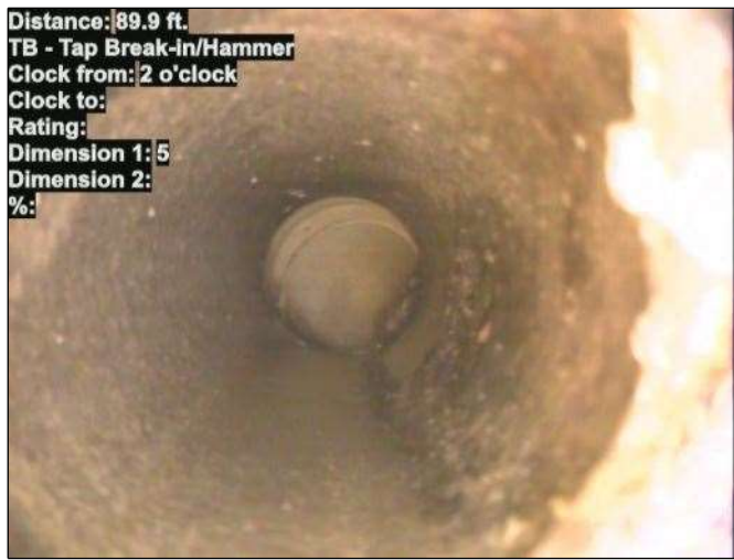
Photo: 15_046-15_047-20230725-092501.JPG At: 89.9 ft. 2/. TB - Tap Break-in/Hammer Joint: No
