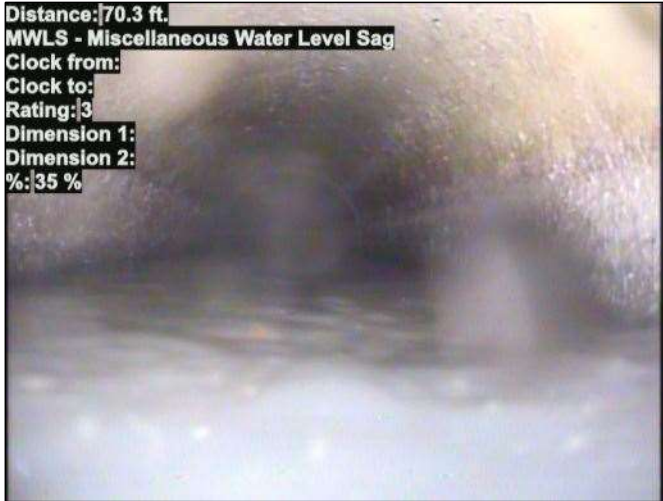
Photo: 15_059-15_060-20230804-085304.JPG At: 70.3 ft. MWLS - Miscellaneous Water Level Sag Joint: No 35 %
