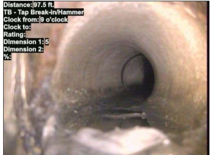
Photo: 15_077-15_078-20230801-071731.JPG At: 97.5 ft. 9/. TB - Tap Break-in/Hammer Joint: No
