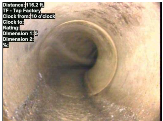
Distance: 116.2 ft. TF - Tap Factory Clock from: 10 o'clock Clock to: Rating: Dimension 1: 5 Dimension 2: %: Photo: 15_045-15_046-20230725-091303.JPG At: 116.2 ft. 10/. TF - Tap Factory Joint: No
