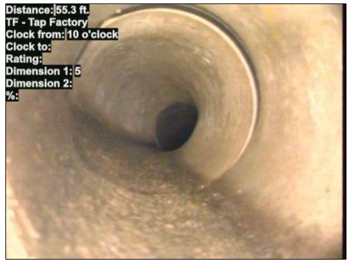
Distance: 55.3 ft. TF - Tap Factory Clock from: 10 o'clock Clock to: Rating: Dimension 1: 5 Dimension 2: %: Photo: 15_045-15_046-20230725-090932.JPG At: 55.3 ft. 10/. TF - Tap Factory Joint: No
