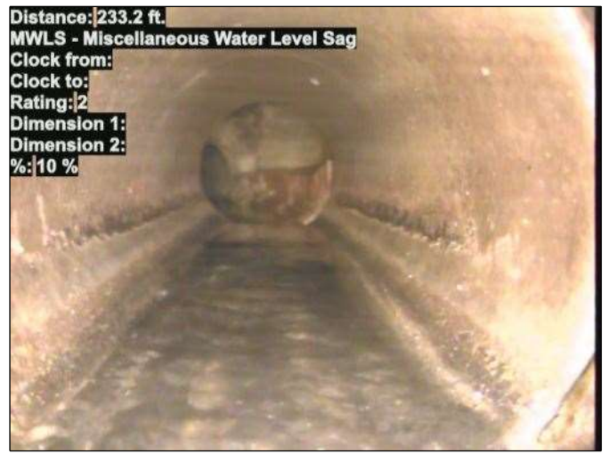
Distance: 233.2 ft. MWLS - Miscellaneous Water Level Sag Clock from: Clock to: Rating: 2 Dimension 1: Dimension 2: %: 10 % Photo: 15_074-15_075-20230726-085126.JPG At: 233.2 ft. MWLS - Miscellaneous Water Level Sag Joint: No 10 %
