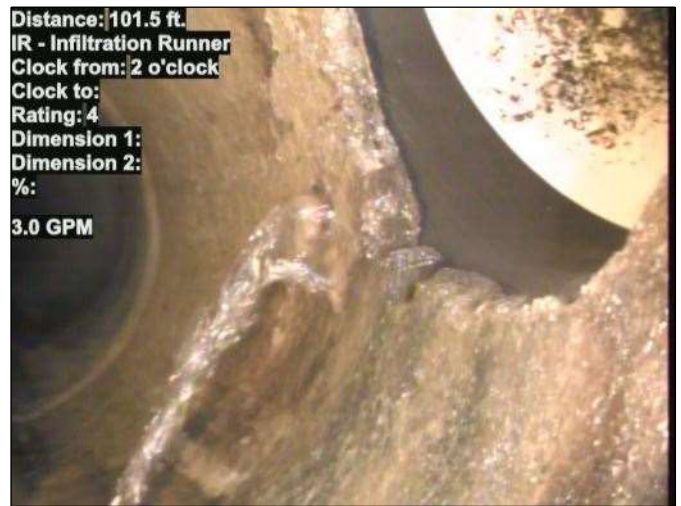
Distance: 101.5 ft. IR - Infiltration Runner Clock from: 2 o'clock Clock to: Rating: 4 Dimension 1: Dimension 2: %: 3.0 GPM Photo: 15_045-15_046-20230725-091147.JPG At: 101.5 ft. 2/. IR - Infiltration Runner Joint: No 3.0 GPM
