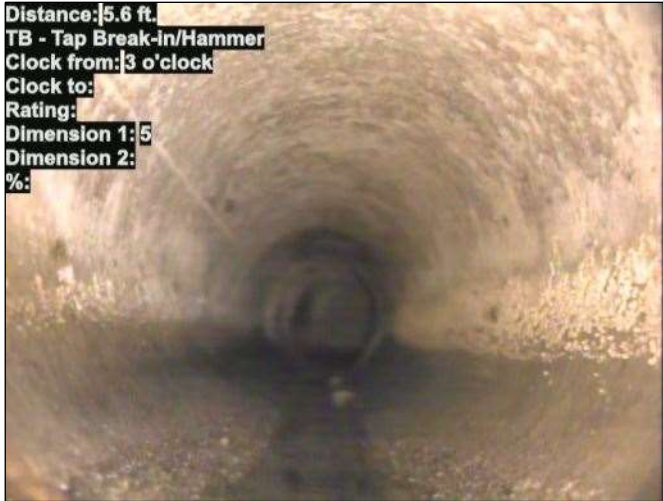
Photo: 15_077-15_078-20230801-071416.JPG At: 5.6 ft. 3/. TB - Tap Break-in/Hammer Joint: No
