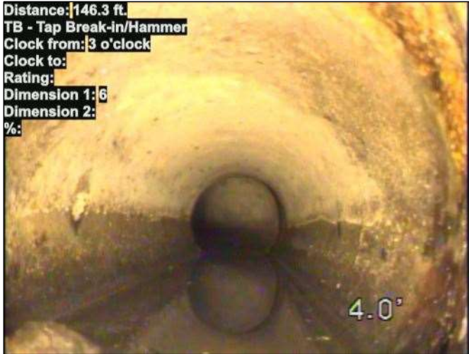
Photo: STUB-15_012-20230807-120402.JPG At: 146.3 ft. 3/. TB - Tap Break-in/Hammer Joint: No
