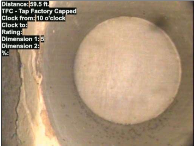
Photo: 15_046-15_047-20230725-092159.JPG At: 59.5 ft. 10/. TFC - Tap Factory Capped Joint: No
