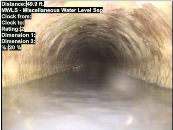
Photo: 15_043-15_058-20230804-071848.JPG At: 49.9 ft. MWLS - Miscellaneous Water Level Sag Joint: No 20 %
