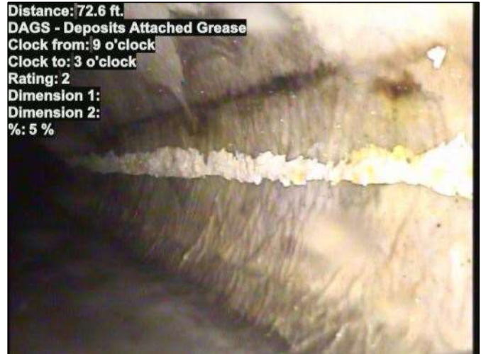
Photo: 15_043-15_058-20230804-071949.JPG At: 72.6 ft. 9/3 DABS - Deposits Attached Grease Joint: No 5 %
