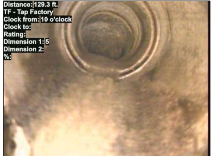
Distance: 129.3 ft. TF - Tap Factory Clock from: 10 o'clock Clock to: Rating: Dimension 1: 5 Dimension 2: %: Photo: 15_072-15_074-20230726-083321.JPG At: 129.3 ft. 10/. TF - Tap Factory Joint: No
