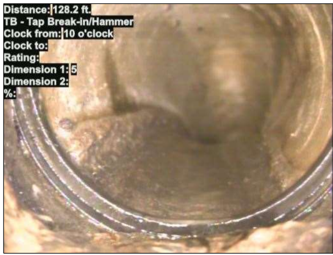
Distance: 128.2 ft. TB - Tap Break-in/Hammer Clock from: 10 o'clock Clock to: Rating: Dimension 1: 5 Dimension 2: %: Photo: 15_016-15_017-20230724-140737.JPG At: 128.2 ft. 10/. TB - Tap Break-in/Hammer Joint: No
