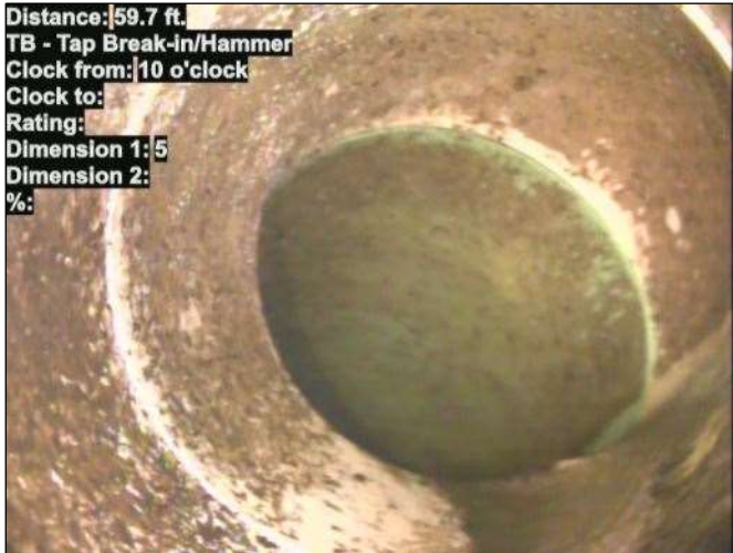
Photo: 15_017-15_018-20230724-150542.JPG At: 59.7 ft. 10/. TB - Tap Break-in/Hammer Joint: No
