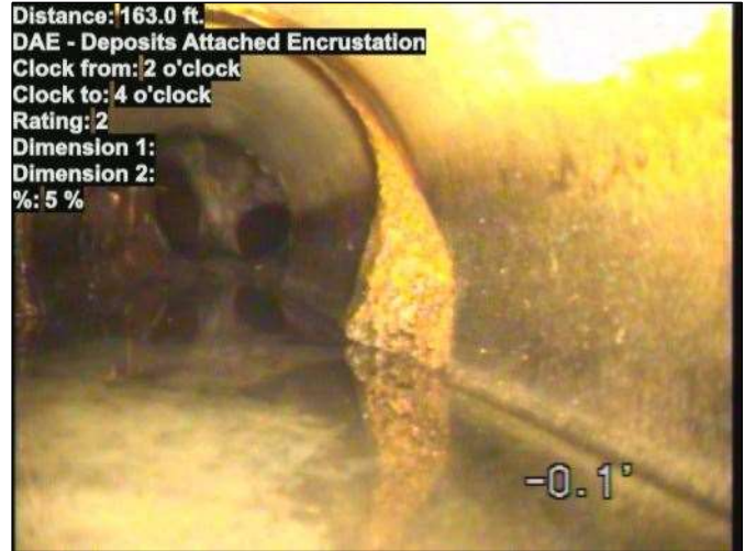
Photo: 15_007-15_006-20230807-105737.JPG At: 163 ft. 2/4 DAE - Deposits Attached Encrustation Joint: No 5 %
