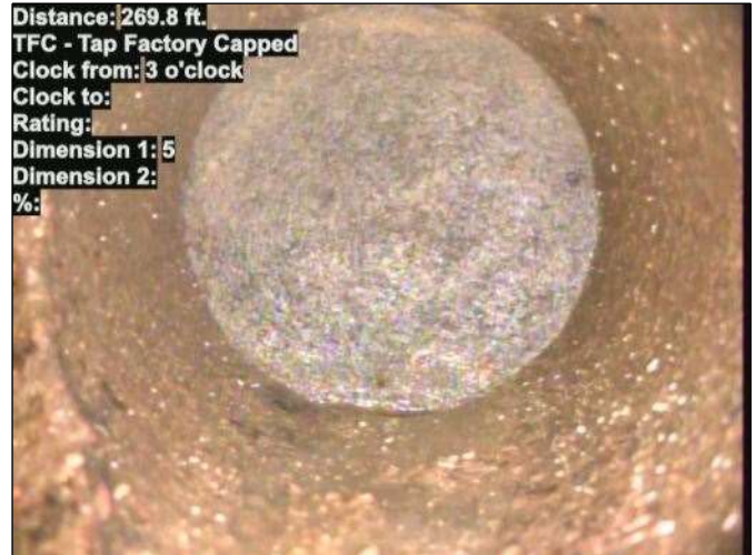
Photo: 15_001-15_002-20230725-122554.JPG At: 269.8 ft. 3/. TFC - Tap Factory Capped Joint: No
