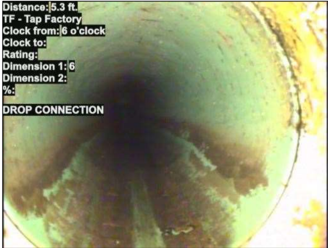
Photo: CLEANOUT-15_108-20230807-093006.JPG At: 5.3 ft. 6/. TF - Tap Factory Joint: No DROP CONNECTION
