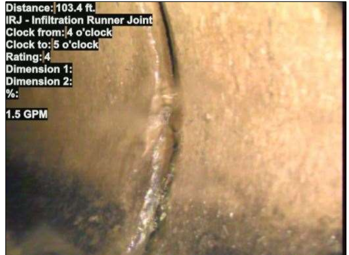
Photo: 15_022-15_023-20230724-154742.JPG At: 103.4 ft. 4/5 IRJ - Infiltration Runner Joint Joint: Yes 1.5 GPM
