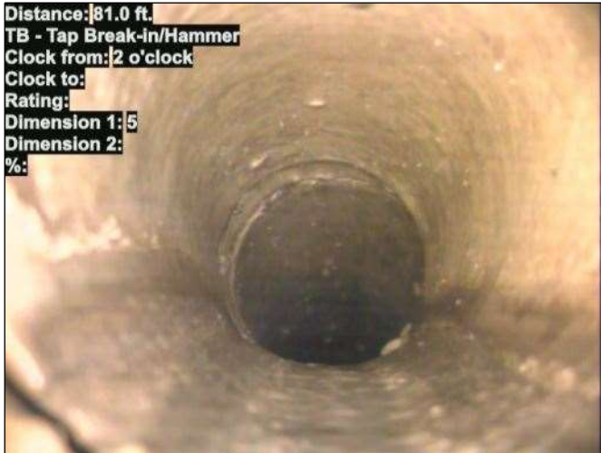
Photo: 15_016-15_017-20230724-140515.JPG At: 81 ft. 2/. TB - Tap Break-in/Hammer Joint: No
