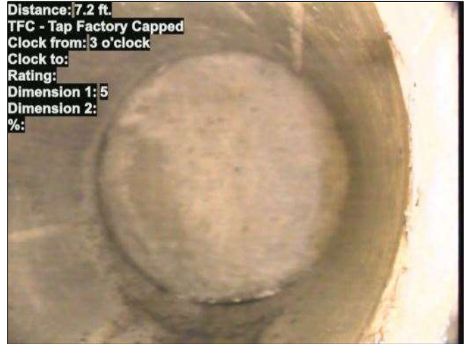
Photo: 15_047-15_048-20230725-093300.JPG At: 7.2 ft. 3/. TFC - Tap Factory Capped Joint: No
