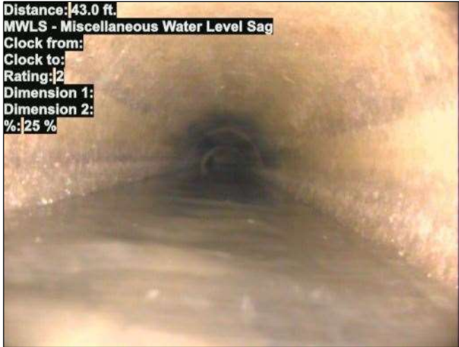
Photo: 15_041-15_042-20230801-123857.JPG At: 43 ft. MWLS - Miscellaneous Water Level Sag Joint: No 25 %
