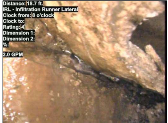
Photo: 15_045-15_046-20230725-090354.JPG At: 18.7 ft. 8/. IRL - Infiltration Runner Lateral Joint: No 2.0 GPM
