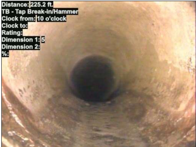
Photo: 15_009A-15_006-20230726-105140.JPG At: 225.2 ft. 10/. TB - Tap Break-in/Hammer Joint: No
