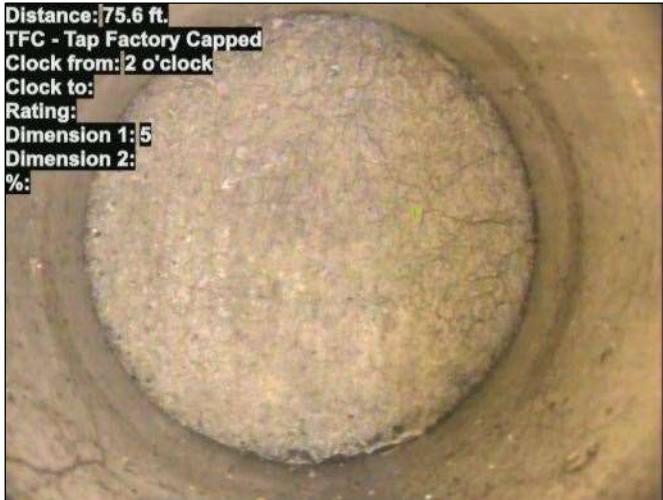
Photo: 15_029-15_030-20230724-164310.JPG At: 75.6 ft. 2/. TFC - Tap Factory Capped Joint: No
