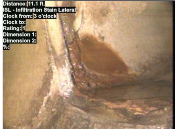
Photo: 15_075-15_076-20230726-085724.JPG At: 11.1 ft. 3/. ISL - Infiltration Stain Lateral Joint: No
