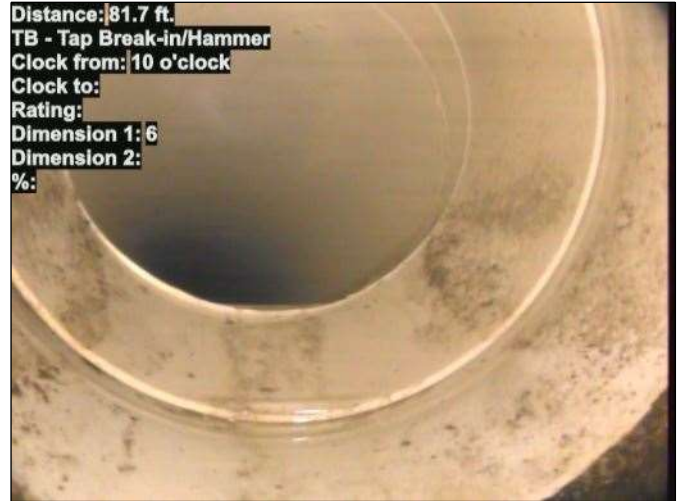
Photo: 15_009A-15_006-20230726-104722.JPG At: 81.7 ft. 10/. TB - Tap Break-in/Hammer Joint: No
