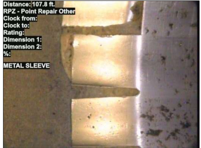
Photo: 15_070-15_071-20230726-081401.JPG At: 107.8 ft. RPZ - Point Repair Other Joint: No METAL SLEEVE
