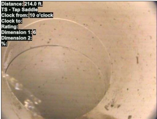
Distance: 214.0 ft. TS - Tap Saddle Clock from: 10 o'clock Clock to: Rating: Dimension 1: 6 Dimension 2: %: Photo: 15_006-15_005-20230726-110754.JPG At: 214 ft. 10/. TS - Tap Saddle Joint: No
