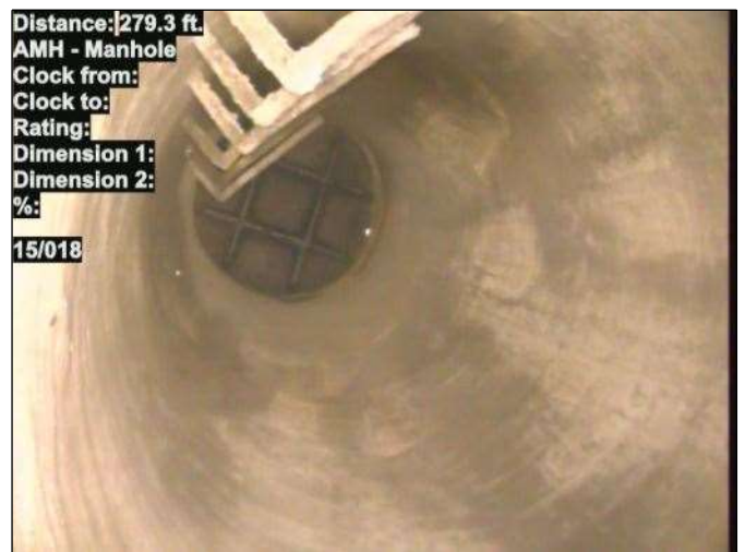
Distance: 279.3 ft. AMH - Manhole Clock from: Clock to: Rating: 5 Dimension 1: Dimension 2: %: 15/018 Photo: 15_019-15_018-20230721-115327.JPG At: 279.3 ft. AMH - Manhole Joint: No 15/018
