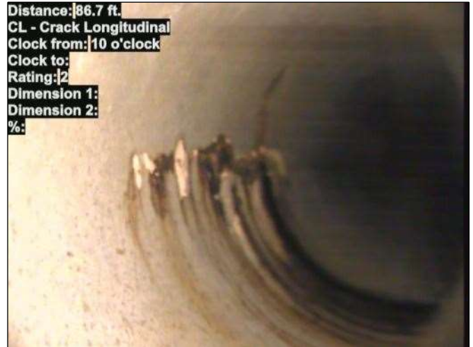
Photo: 15_014-15_015-20230724-143819.JPG At: 86.7 ft. 10/. CL - Crack Longitudinal Joint: No
