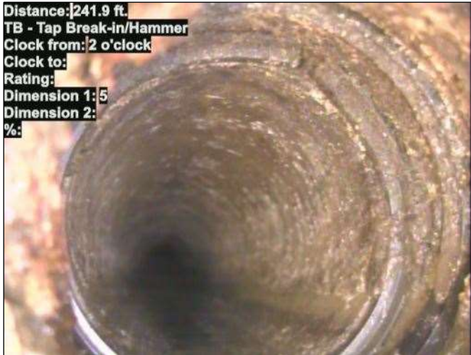
Photo: 15_002-15_003-20230725-113040_1.JPG At: 241.9 ft. 2/. TB - Tap Break-in/Hammer Joint: No
