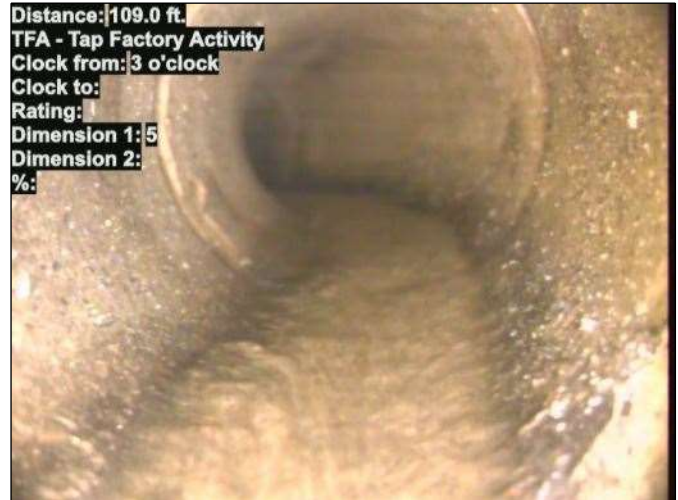
Photo: 15_042-15_043-20230801-130703.JPG At: 109 ft. 3/. TFA - Tap Factory Activity Joint: No
