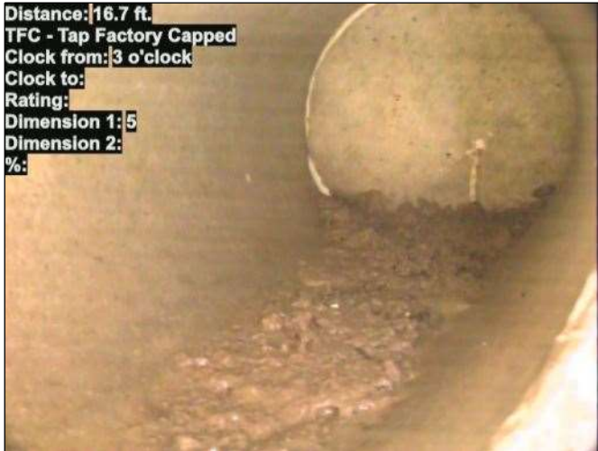
Photo: 15_075-15_076-20230726-085822.JPG At: 16.7 ft. 3/. TFC - Tap Factory Capped Joint: No
