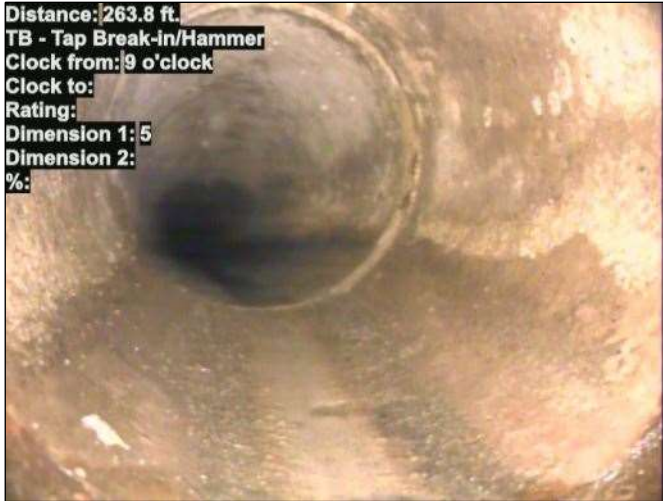
Photo: 15_012-15_011-20230726-101745.JPG At: 263.8 ft. 9/. TB - Tap Break-in/Hammer Joint: No
