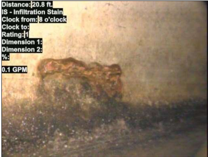
Photo: 15_076-15_077-20230726-091027.JPG At: 20.8 ft. 8/. IS - Infiltration Stain Joint: No 0.1 GPM
