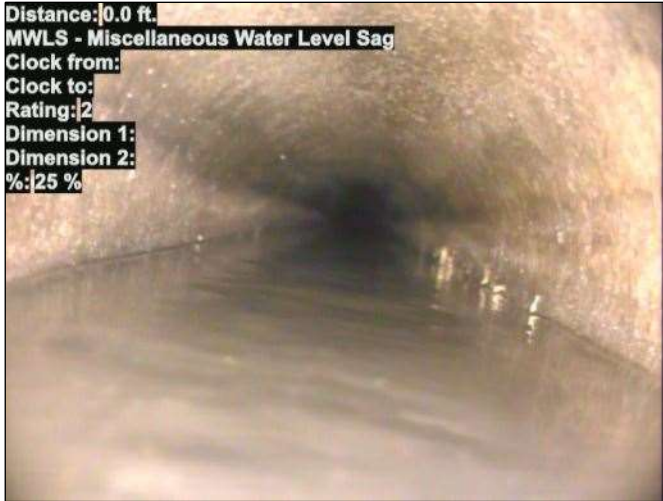
Photo: 15_034-15_036-20230801-105433.JPG At: 0 ft. MWLS - Miscellaneous Water Level Sag Joint: No 25 %
