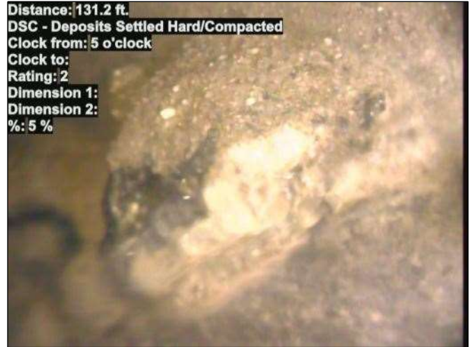
Photo: 15_078-15_061-20230801-082338.JPG At: 131.2 ft. 5/. DSC - Deposits Settled Hard/Compacted Joint: No 5 %
