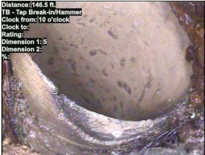
Distance: 146.5 ft. TB - Tap Break-in/Hammer Clock from: 10 o'clock Clock to: Rating: Dimension 1: 5 Dimension 2: %: Photo: 15_092-15_062-20230804-112952.JPG At: 146.5 ft. 10/. TB - Tap Break-in/Hammer Joint: No
