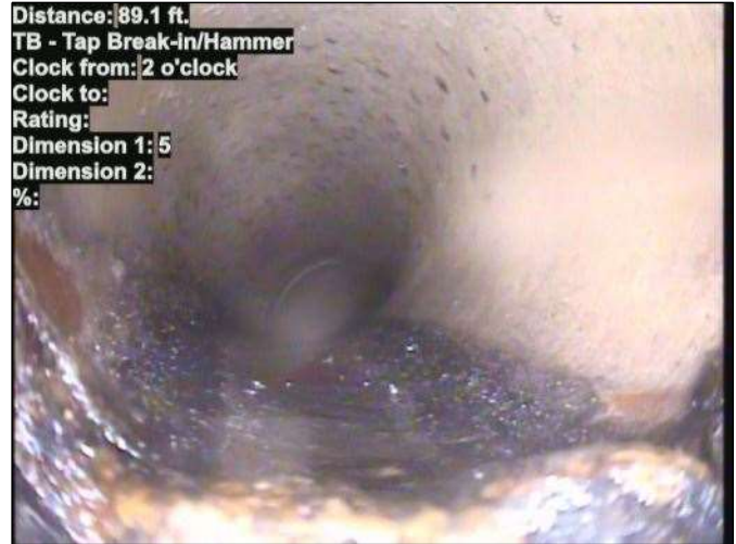
Distance: 89.1 ft. TB - Tap Break-in/Hammer Clock from: 2 o'clock Clock to: Rating: Dimension 1: 5 Dimension 2: %: Photo: 15_092-15_062-20230804-112433.JPG At: 89.1 ft. 2/. TB - Tap Break-in/Hammer Joint: No
