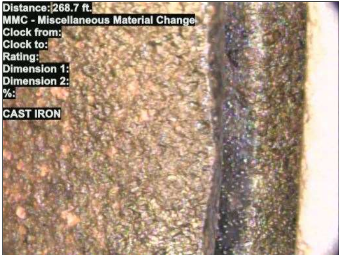
Photo: 15_001-15_002-20230725-122534.JPG At: 268.7 ft. MMC - Miscellaneous Material Change Joint: No CAST IRON
