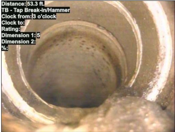
Photo: 15_018-15_025-20230801-095000.JPG At: 53.3 ft. 3/. TB - Tap Break-in/Hammer Joint: No
