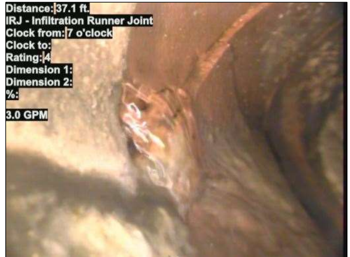
Photo: 15_039-15_040-20230724-124448.JPG At: 37.1 ft. 7/. IRJ - Infiltration Runner Joint Joint: Yes 3.0 GPM
