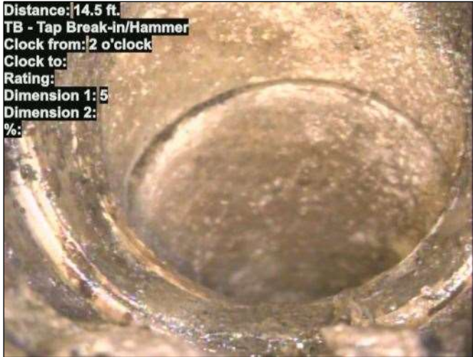
Photo: 15_030-15_031-20230724-165146.JPG At: 14.5 ft. 2/. TB - Tap Break-in/Hammer Joint: No
