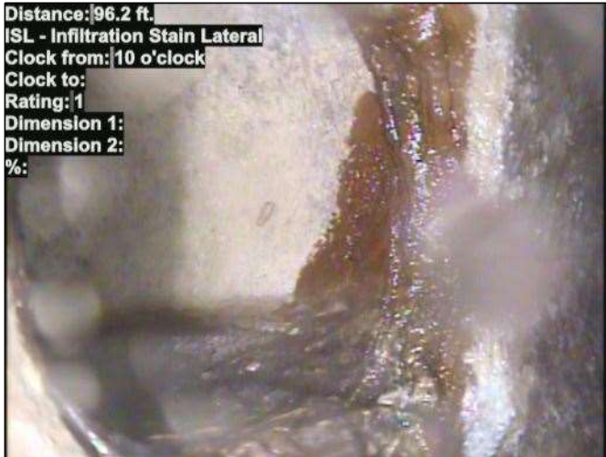
Photo: 15_059-15_060-20230804-085444.JPG At: 96.2 ft. 10/. ISL - Infiltration Stain Lateral Joint: No
