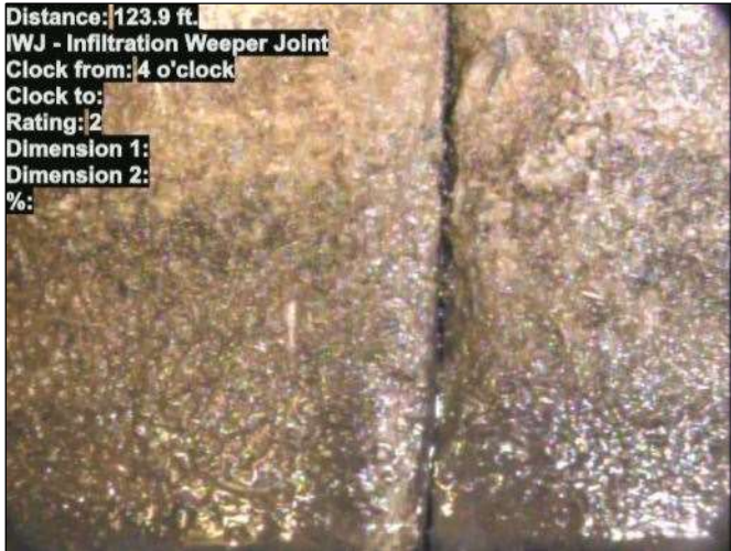
Photo: 15_005-15_018-20230801-091813.JPG At: 123.9 ft. 4/. IWJ - Infiltration Weeper Joint Joint: Yes
