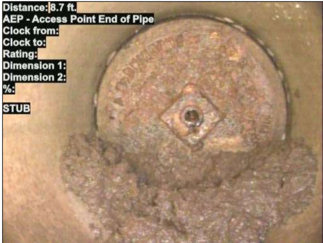
Photo: STUB-15_070-20230726-094435.JPG At: 8.7 ft. AEP - Access Point End of Pipe Joint: No STUB
