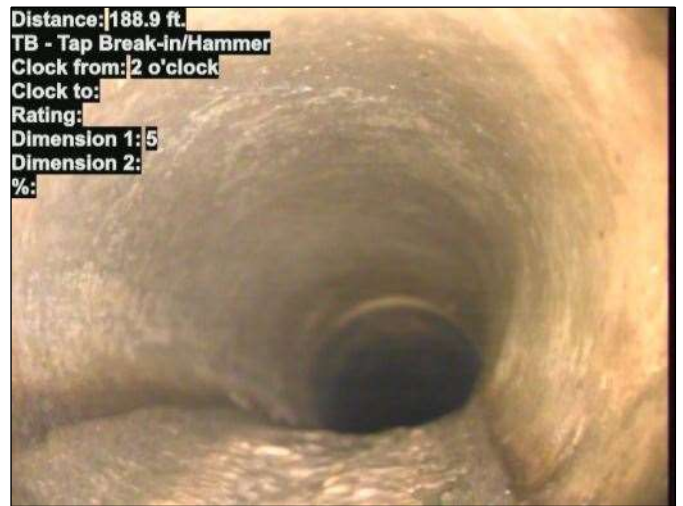
Distance: 188.9 ft. TB - Tap Break-in/Hammer Clock from: 2 o'clock Clock to: Rating: Dimension 1: 5 Dimension 2: %: Photo: 15_014-15_015-20230724-144333.JPG At: 188.9 ft. 2/. TB - Tap Break-in/Hammer Joint: No
