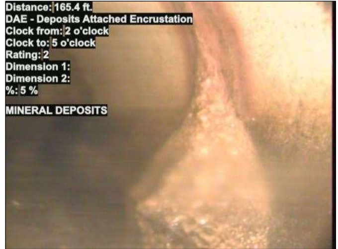
Photo: 15_007-15_006-20230726-125205.JPG At: 165.4 ft. 2/5 DAE - Deposits Attached Encrustation Joint: No 5 % MINERAL DEPOSITS
