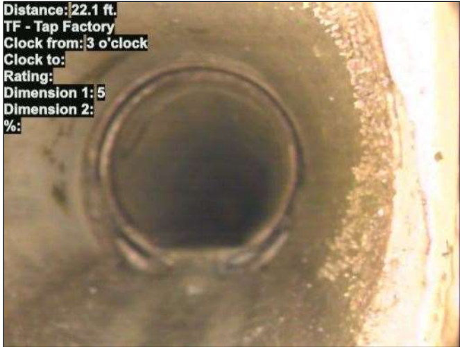
Distance: 22.1 ft. TF - Tap Factory Clock from: 3 o'clock Clock to: Rating: Dimension 1: 5 Dimension 2: %: Photo: 15_072-15_074-20230726-082832.JPG At: 22.1 ft. 3/. TF - Tap Factory Joint: No
