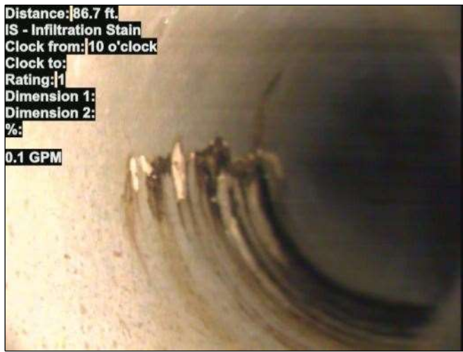
Distance: 86.7 ft. IS - Infiltration Stain Clock from: 10 o'clock Clock to: Rating: 1 Dimension 1: Dimension 2: %: 0.1 GPM Photo: 15_014-15_015-20230724-143825.JPG At: 86.7 ft. 10/. IS - Infiltration Stain Joint: No 0.1 GPM
