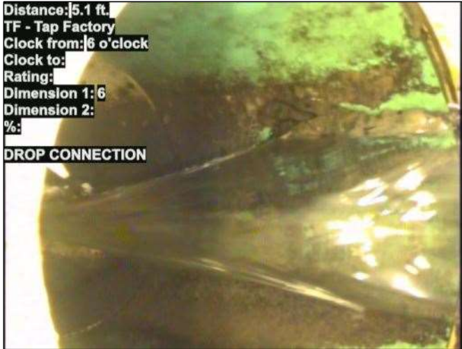
Photo: CLEANOUT-15_109-20230807-085936.JPG At: 5.1 ft. 6/. TF - Tap Factory Joint: No DROP CONNECTION
