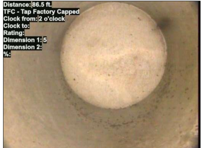
Photo: 15_046-15_047-20230725-092418.JPG At: 86.5 ft. 2/. TFC - Tap Factory Capped Joint: No
