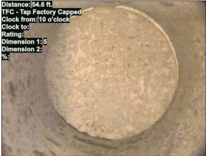
Photo: 15_038-15_039-20230724-123416.JPG At: 54.6 ft. 10/. TFC - Tap Factory Capped Joint: No
