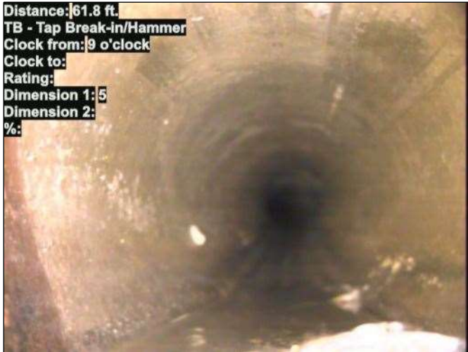
Photo: 15_046-15_047-20230725-092314.JPG At: 61.8 ft. 9/. TB - Tap Break-in/Hammer Joint: No
