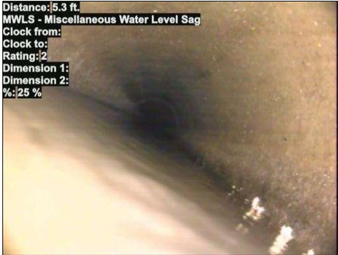
Photo: 15_040-15_041-20230801-123023.JPG At: 5.3 ft. MWLS - Miscellaneous Water Level Sag Joint: No 25 %
