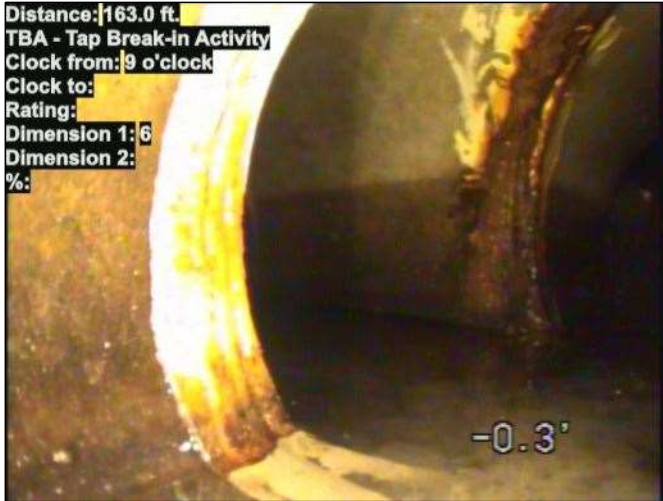
Photo: 15_007-15_006-20230807-105714.JPG At: 163 ft. 9/. TBA - Tap Break-in Activity Joint: No
