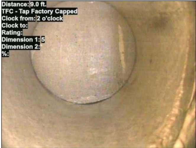
Photo: 15_044-15_045-20230725-085452.JPG At: 9 ft. 2/. TFC - Tap Factory Capped Joint: No
