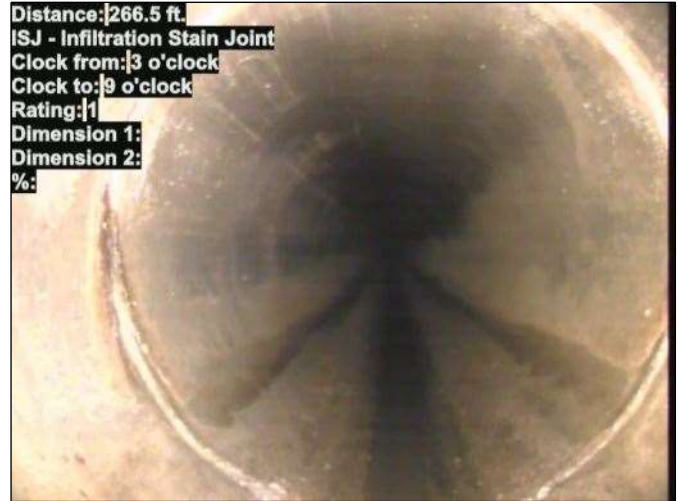
Photo: 15_012-15_011-20230726-101829.JPG At: 266.5 ft. 3/9 ISJ - Infiltration Stain Joint Joint: Yes
