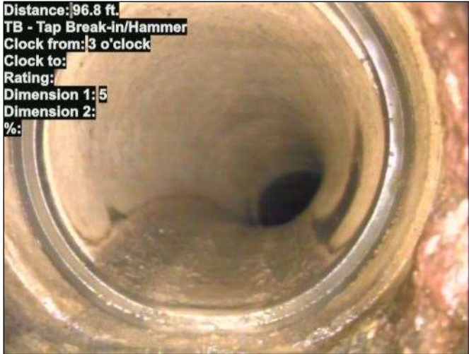
Photo: 15_003-15_004-20230725-113833.JPG At: 96.8 ft. 3/. TB - Tap Break-in/Hammer Joint: No
