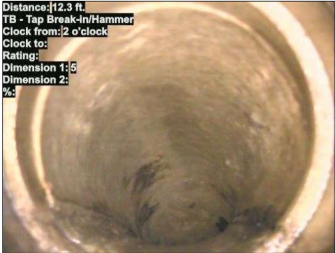
Photo: 15_016-15_017-20230724-140230.JPG At: 12.3 ft. 2/. TB - Tap Break-in/Hammer Joint: No
