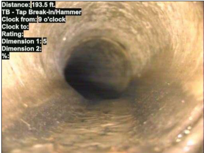
Photo: 15_015-15_016-20230724-135701.JPG At: 193.5 ft. 9/. TB - Tap Break-in/Hammer Joint: No
