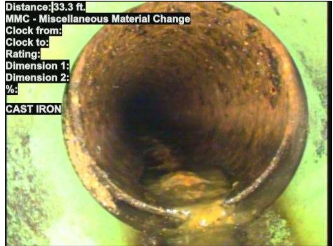
Photo: CLEANOUT-15_111-20230807-094759.JPG At: 33.3 ft. MMC - Miscellaneous Material Change Joint: No CAST IRON
