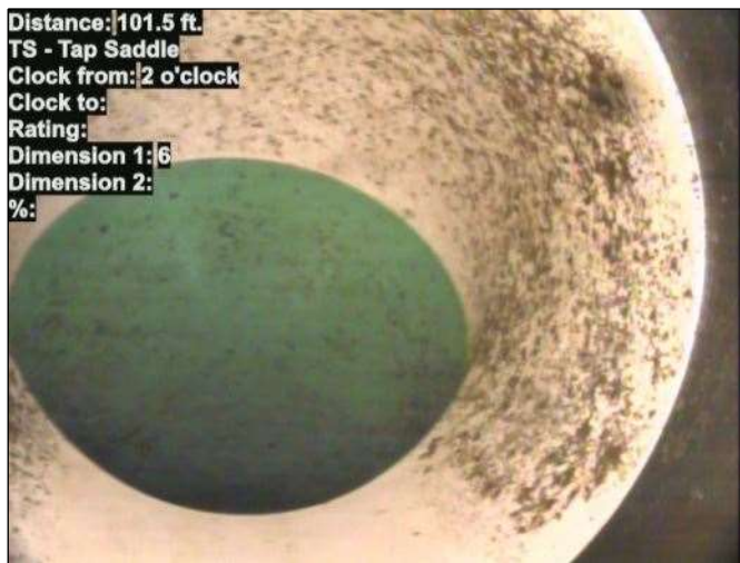
Distance: 101.5 ft. TS - Tap Saddle Clock from: 2 o'clock Clock to: Rating: Dimension 1: 6 Dimension 2: %: Photo: 15_045-15_046-20230725-091130.JPG At: 101.5 ft. 2/. TS - Tap Saddle Joint: No
