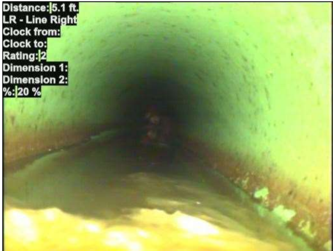
Photo: CLEANOUT-15_109-20230807-090026.JPG At: 5.1 ft. LR - Line Right Joint: No 20 %
