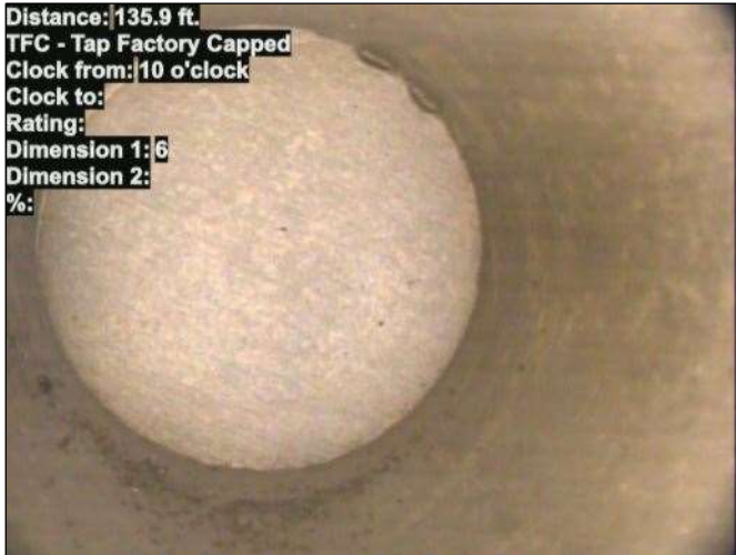
Photo: 15_013-15_014-20230725-125150.JPG At: 135.9 ft. 10/. TFC - Tap Factory Capped Joint: No
