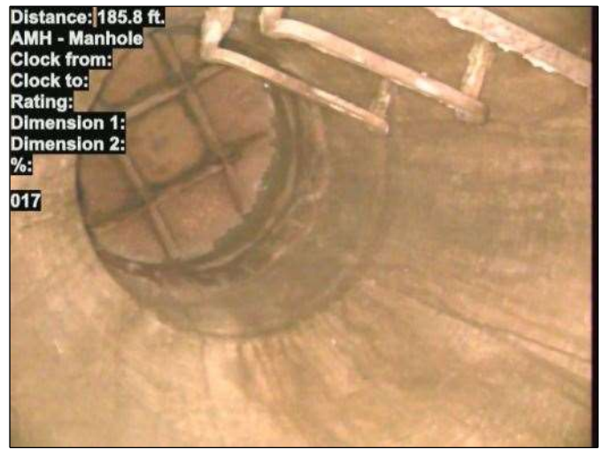
Distance: 185.8 ft. AMH - Manhole Clock from: Clock to: Rating: Dimension 1: Dimension 2: %: 017 Photo: 15_016-15_017-20230724-141048.JPG At: 185.8 ft. AMH - Manhole Joint: No 017
