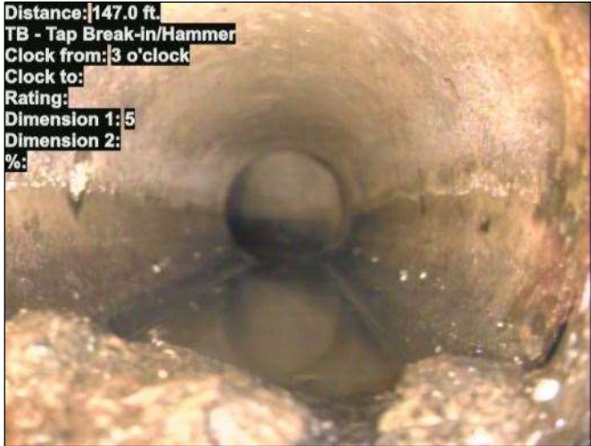
Photo: STUB-15_012-20230726-113650.JPG At: 147 ft. 3/. TB - Tap Break-in/Hammer Joint: No
