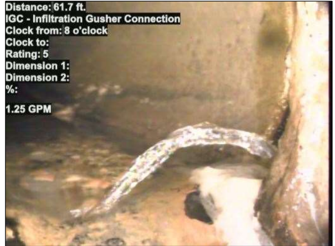
Photo: 15_046-15_047-20230725-092224.JPG At: 61.7 ft. 8/. IGC - Infiltration Gusher Connection Joint: No 1.25 GPM
