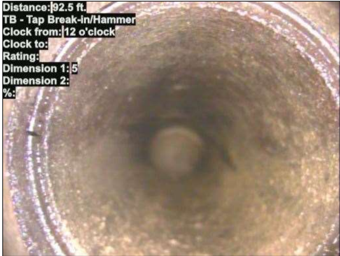
Photo: 15_036-15_040-20230801-111753.JPG At: 92.5 ft. 12/. TB - Tap Break-in/Hammer Joint: No
