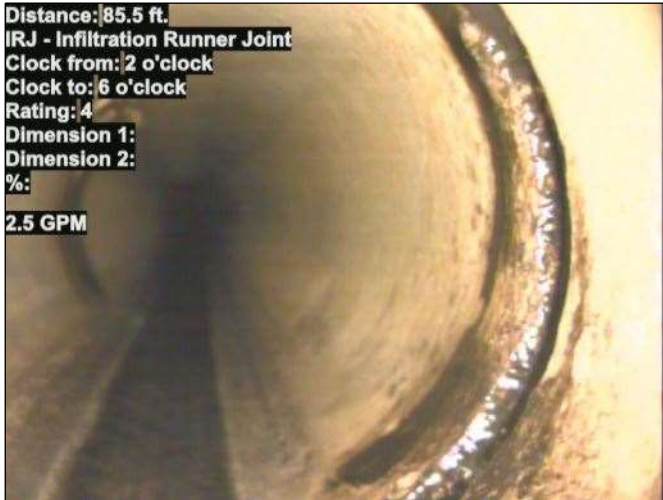
Photo: 15_014-15_015-20230724-143735.JPG At: 85.5 ft. 2/6 IRJ - Infiltration Runner Joint Joint: Yes 2.5 GPM
