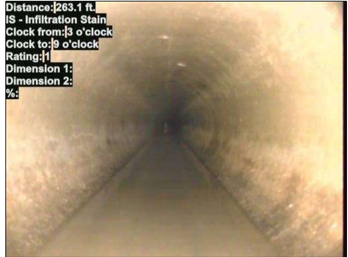
Photo: 15_004-15_005-20230725-121258.JPG At: 264 ft. 3/9 IS - Infiltration Stain Joint: No
