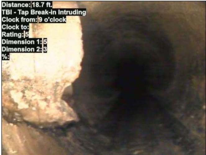
Photo: 15_045-15_046-20230725-090324_1.JPG At: 18.7 ft. 9/. TBI - Tap Break-in Intruding Joint: No
