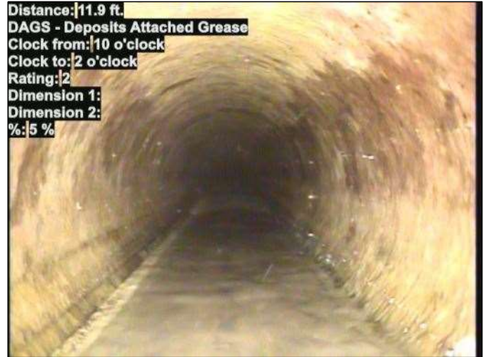
Photo: 15_043-15_058-20230804-071723.JPG At: 11.9 ft. 10/2 DABS - Deposits Attached Grease Joint: No 5 %
