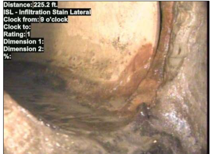
Photo: 15_009A-15_006-20230726-105205.JPG At: 225.2 ft. 9/. ISL - Infiltration Stain Lateral Joint: No
