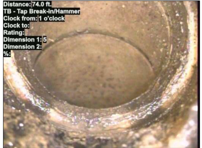
Photo: 15_034-15_036-20230801-105708.JPG At: 74 ft. 1/. TB - Tap Break-in/Hammer Joint: No
