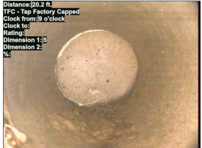
Photo: 15_075-15_076-20230726-085906.JPG At: 20.2 ft. 9/. TFC - Tap Factory Capped Joint: No
