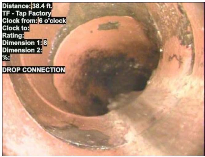
Distance: 38.4 ft. TF - Tap Factory Clock from: 6 o'clock Clock to: Rating: Dimension 1: 8 Dimension 2: %: Photo: 15_039-15_040-20230724-124611.JPG At: 38.4 ft. 6/. TF - Tap Factory Joint: No DROP CONNECTION
