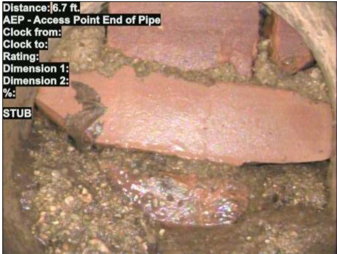
Photo: STUB-15_013-20230725-130223.JPG At: 6.7 ft. AEP - Access Point End of Pipe Joint: No STUB
