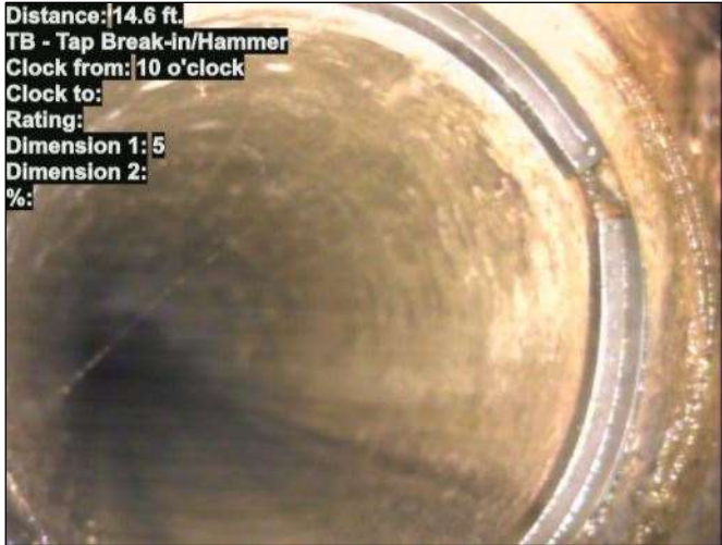
Photo: 15_015-15_016-20230724-135227.JPG At: 14.6 ft. 10/. TB - Tap Break-in/Hammer Joint: No
