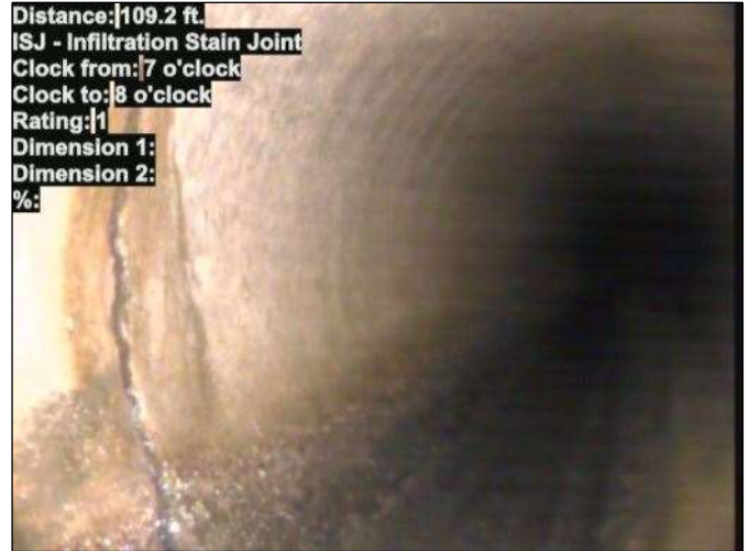
Photo: 15_013-15_014-20230725-125038.JPG At: 109.2 ft. 7/8 ISJ - Infiltration Stain Joint Joint: Yes
