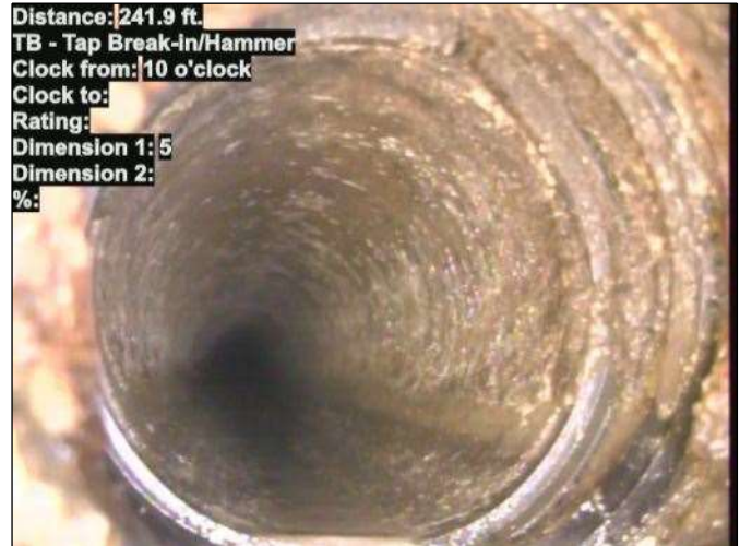
Photo: 15_002-15_003-20230725-113040.JPG At: 241.9 ft. 2/. TB - Tap Break-in/Hammer Joint: No
