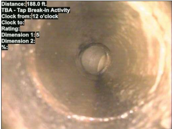
Photo: 15_024-15_033-20230801-101537.JPG At: 188 ft. 12/. TBA - Tap Break-in Activity Joint: No
