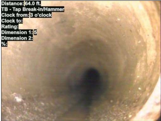
Photo: 15_021-15_022-20230724-153618.JPG At: 64 ft. 3/. TB - Tap Break-in/Hammer Joint: No
