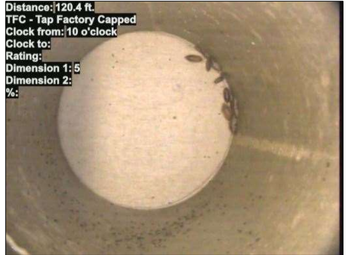
Photo: 15_049-15_050-20230726-063928.JPG At: 120.4 ft. 10/. TFC - Tap Factory Capped Joint: No
