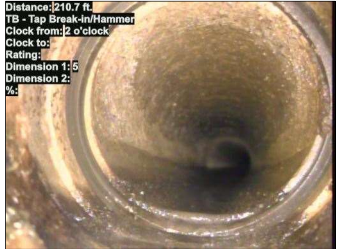
Photo: 15_002-15_003-20230725-112822.JPG At: 210.7 ft. 2/. TB - Tap Break-in/Hammer Joint: No
