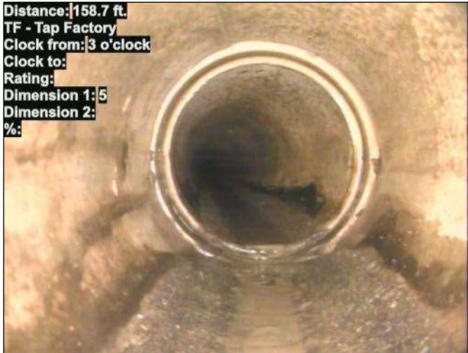
Distance: 158.7 ft. TF - Tap Factory Clock from: 3 o'clock Clock to: Rating: Dimension 1: 5 Dimension 2: %: Photo: 15_072-15_074-20230726-083440.JPG At: 158.7 ft. 3/. TF - Tap Factory Joint: No
