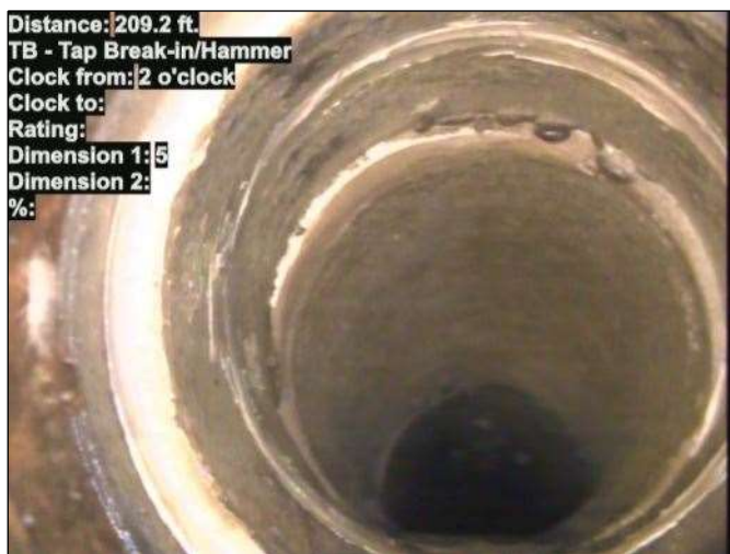
Distance: 209.2 ft. TB - Tap Break-in/Hammer Clock from: 2 o'clock Clock to: Rating: Dimension 1: 5 Dimension 2: %: Photo: 15_014-15_015-20230724-144425.JPG At: 209.2 ft. 2/. TB - Tap Break-in/Hammer Joint: No
