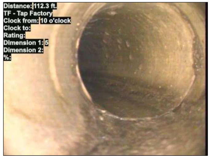
Distance: 112.3 ft. TF - Tap Factory Clock from: 10 o'clock Clock to: Rating: Dimension 1: 5 Dimension 2: %: Photo: 15_014-15_015-20230724-144011.JPG At: 112.3 ft. 10/. TF - Tap Factory Joint: No
