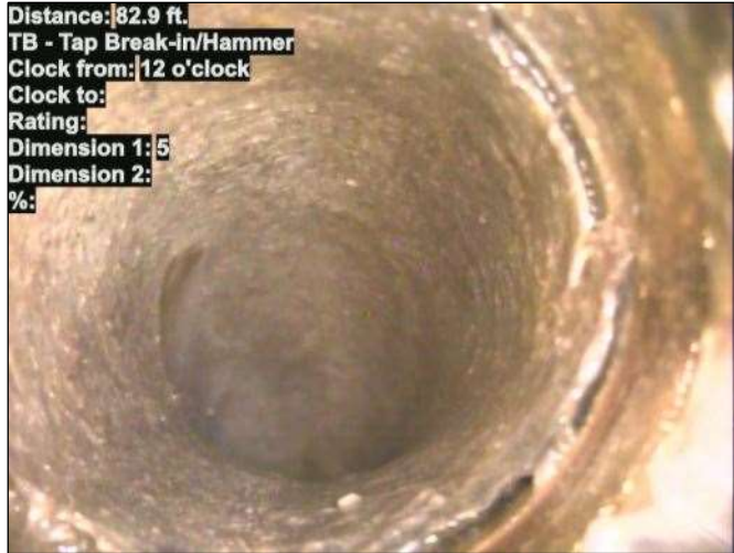
Photo: 15_033-15_034-20230801-104532.JPG At: 82.9 ft. 12/. TB - Tap Break-in/Hammer Joint: No
