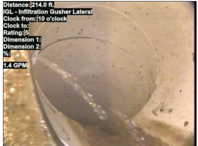
Distance: 214.0 ft. IGL - Infiltration Gusher Lateral Clock from: 10 o'clock Clock to: Rating: 5 Dimension 1: Dimension 2: %: 1.4 GPM Photo: 15_006-15_005-20230726-110809.JPG At: 214 ft. 10/. IGL - Infiltration Gusher Lateral Joint: No 1.4 GPM
