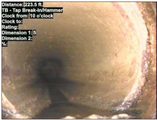
Distance: 223.5 ft. TB - Tap Break-in/Hammer Clock from: 10 o'clock Clock to: Rating: Dimension 1: 5 Dimension 2: %: Photo: 15_074-15_075-20230726-085044.JPG At: 223.5 ft. 10/. TB - Tap Break-in/Hammer Joint: No
