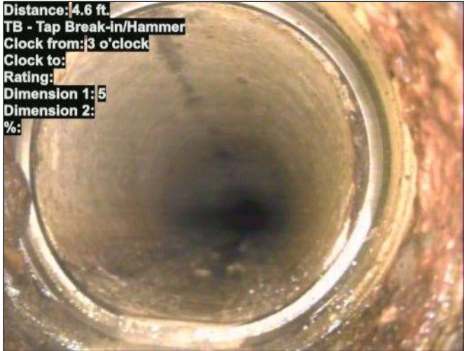
Photo: 15_047-15_048-20230725-093236.JPG At: 4.6 ft. 3/. TB - Tap Break-in/Hammer Joint: No
