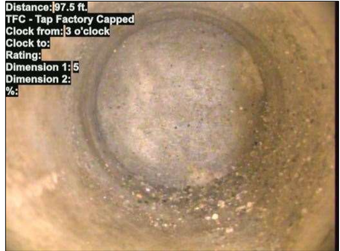
Photo: 15_005-15_018-20230801-091651.JPG At: 97.5 ft. 3/. TFC - Tap Factory Capped Joint: No
