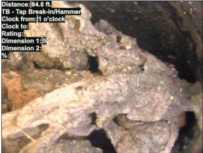
Photo: 15_005-15_018-20230801-091542.JPG At: 84.8 ft. 1/. TB - Tap Break-in/Hammer Joint: No
