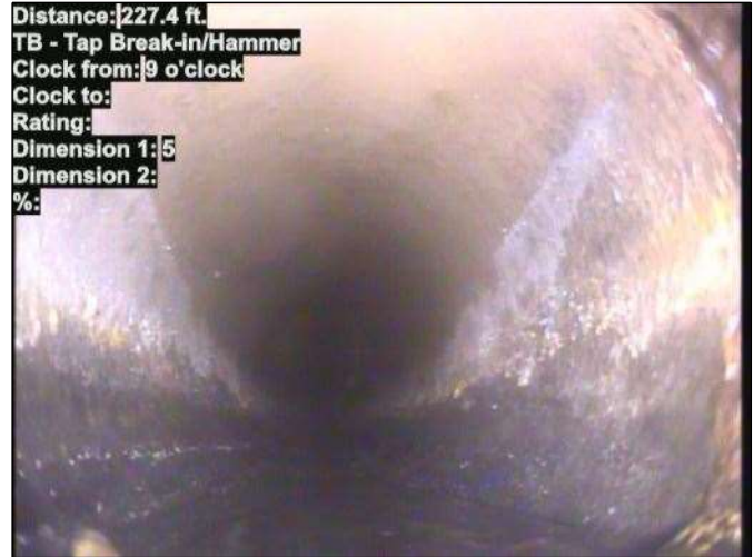
Photo: 15_060-15_061-20230804-102139.JPG At: 227.4 ft. 9/. TB - Tap Break-in/Hammer Joint: No
