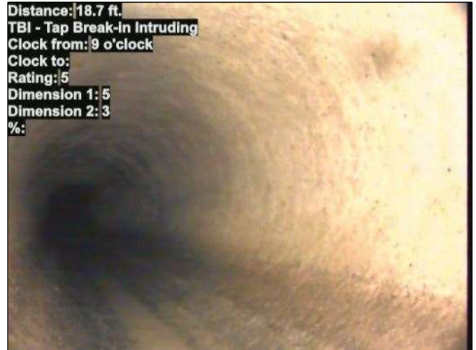
Photo: 15_045-15_046-20230725-090324.JPG At: 18.7 ft. 9/. TBI - Tap Break-in Intruding Joint: No
