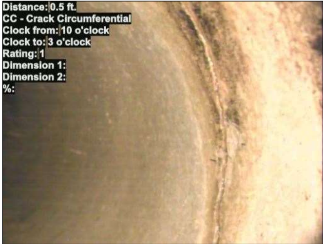
Photo: STUB-15_013-20230725-130325.JPG At: 0.5 ft. 10/3 CC - Crack Circumferential Joint: Yes
