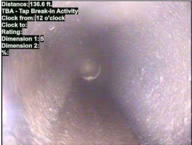
Photo: 15_060-15_061-20230804-101808.JPG At: 136.6 ft. 12/. TBA - Tap Break-in Activity Joint: No
