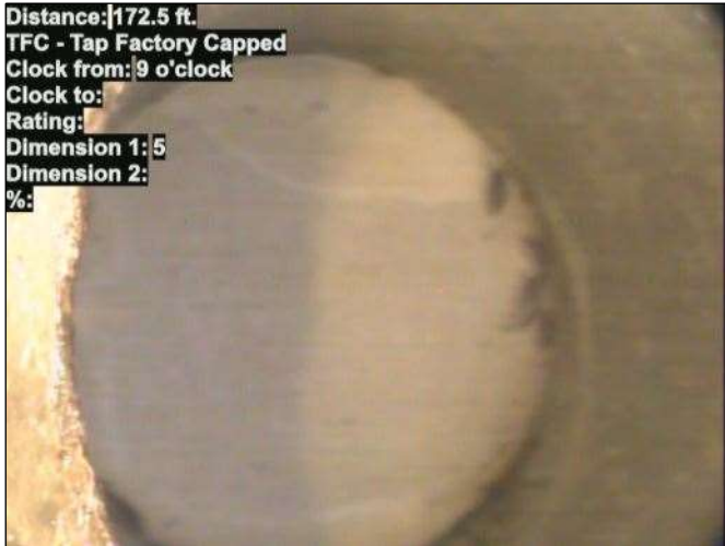
Photo: 15_037-15_038-20230724-122230.JPG At: 172.5 ft. 9/. TFC - Tap Factory Capped Joint: No
