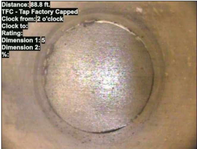
Photo: 15_018-15_025-20230801-095221.JPG At: 88.8 ft. 2/. TFC - Tap Factory Capped Joint: No
