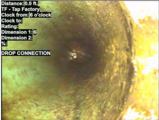
Photo: CLEANOUT-15_111-20230807-094521.JPG At: 0 ft. 6/. TF - Tap Factory Joint: No DROP CONNECTION
