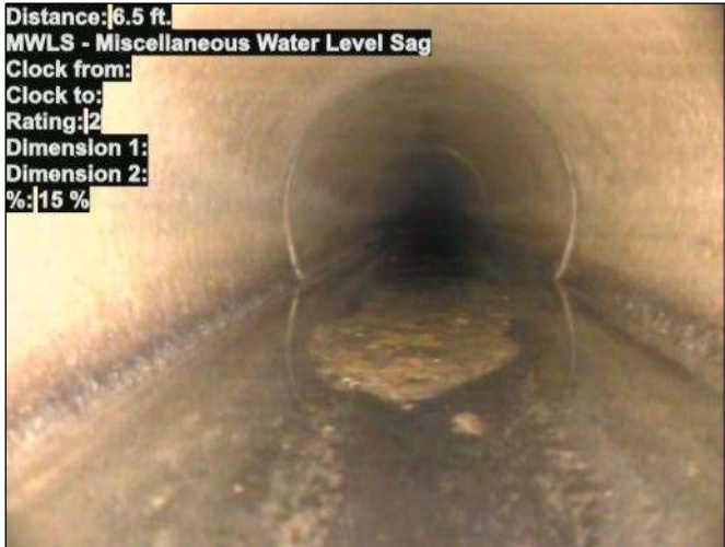
Photo: 15_048-15_033-20230725-103334.JPG At: 6.5 ft. MWLS - Miscellaneous Water Level Sag Joint: No 15 %
