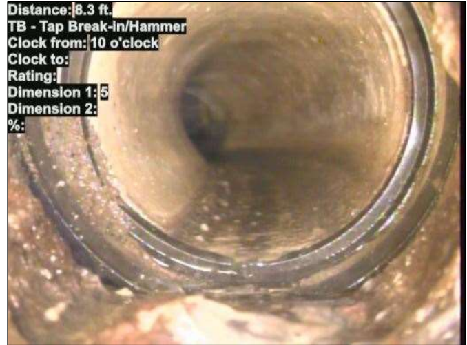
Photo: 15_056-15_057-20230725-074318.JPG At: 8.3 ft. 10/. TB - Tap Break-in/Hammer Joint: No
