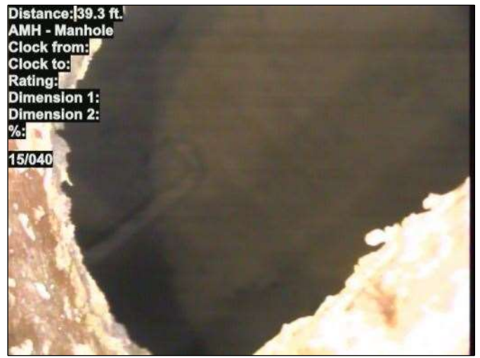
Distance: 39.3 ft. AMH - Manhole Clock from: Clock to: Rating: Dimension 1: Dimension 2: %: 15/040 Photo: 15_039-15_040-20230724-124639.JPG At: 39.3 ft. AMH - Manhole Joint: No 15/040
