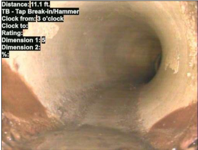
Photo: 15_075-15_076-20230726-085703.JPG At: 11.1 ft. 3/. TB - Tap Break-in/Hammer Joint: No
