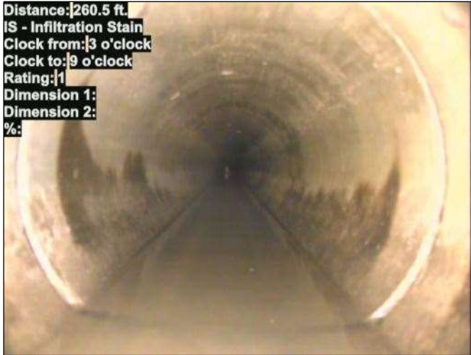
Photo: 15_004-15_005-20230725-115813.JPG At: 260.5 ft. 3/9 IS - Infiltration Stain Joint: No
