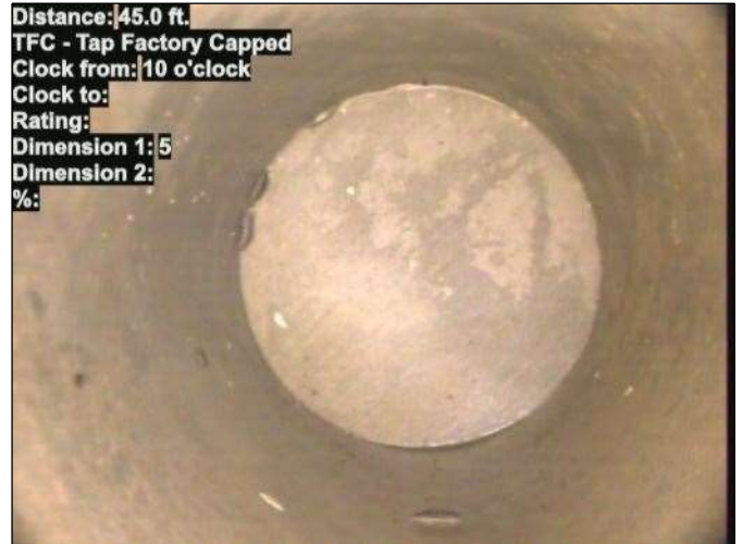
Photo: 15_048-15_033-20230725-103745.JPG At: 45 ft. 10/. TFC - Tap Factory Capped Joint: No
