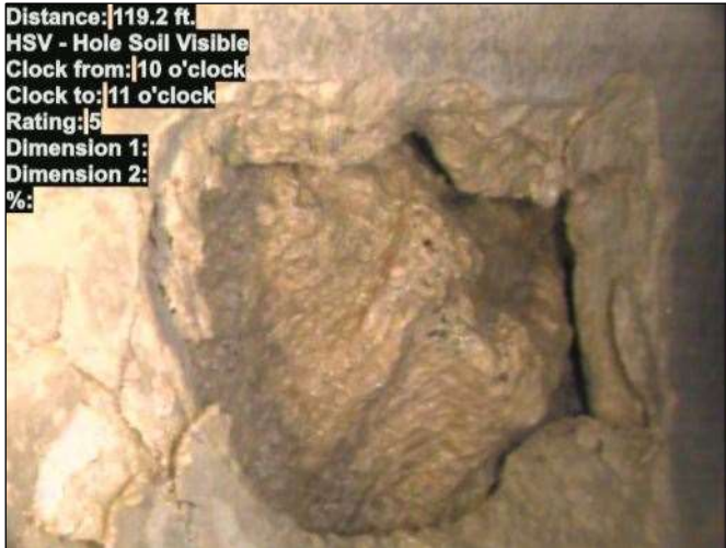
Photo: 15_074-15_075-20230726-084550.JPG At: 119.2 ft. HSV - Hole Soil Visible 10/11 Joint: No
