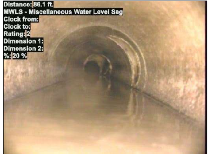
Photo: 15_018-15_025-20230801-095130.JPG At: 86.1 ft. MWLS - Miscellaneous Water Level Sag Joint: No 20 %
