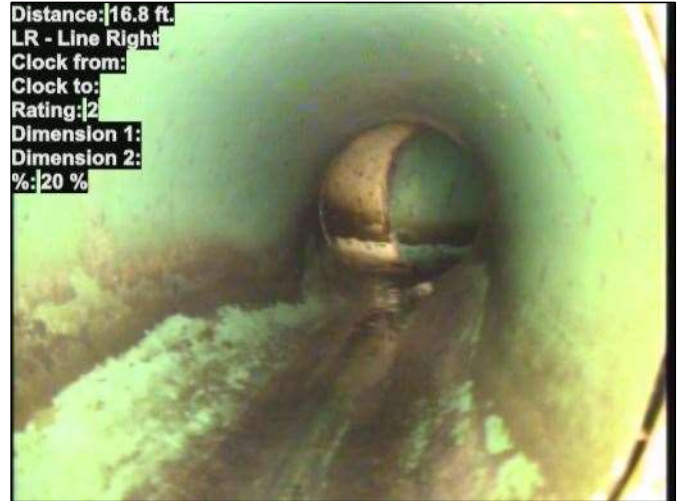
Photo: CLEANOUT-15_108-20230807-093253.JPG At: 16.8 ft. LR - Line Right Joint: No 20 %
