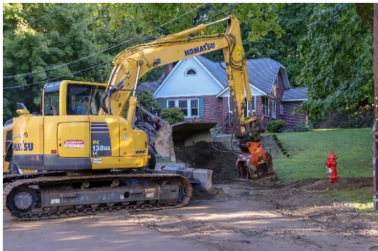
An excavator is making the finishing touches around a newly installed fire hydrant.
