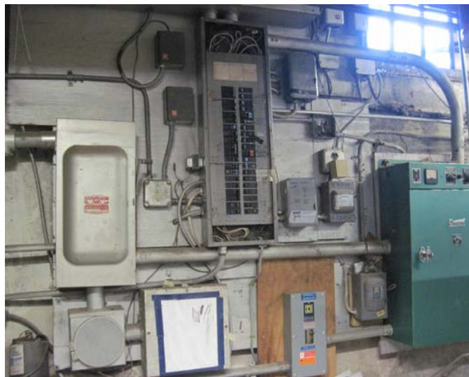
View of the aging electrical distribution equipment and wiring with open-panel electrical load center. All in need of near term modernization.
