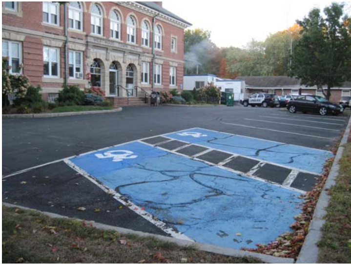
View of the aging front parking lot asphalt surface conditions. Complete resurfacing is planned for 2016.
