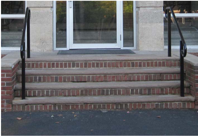
The front steps and adjacent brick planters are in need of near term repointing and brick repair/replacement.
