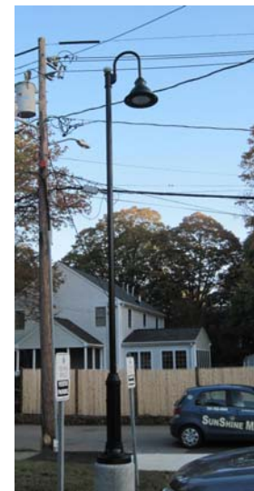
Site lighting is provided by newly installed gooseneck-style LED pole-mounted fixtures.
