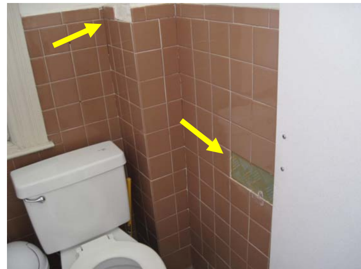
View of damaged and missing tilework within the first floor restroom. In need of near-term updating and remodeling to accessibility standards.
