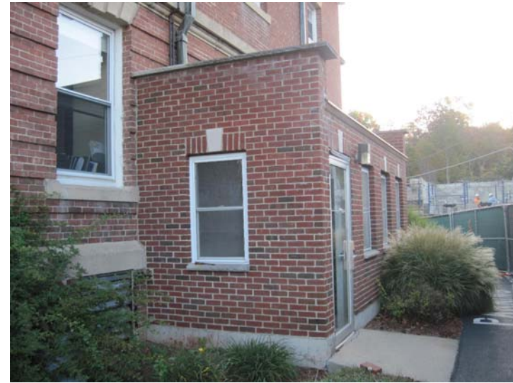
View of the south end-elevation addition, constructed at an unknown later date.
