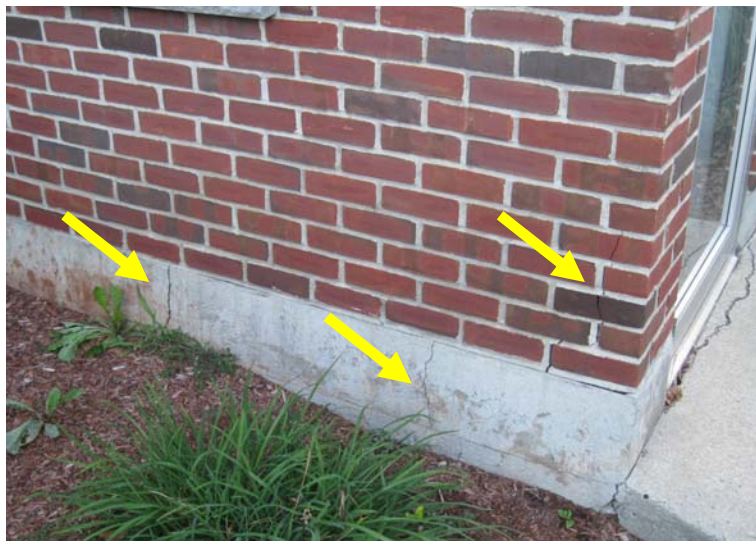
Close-up of visible cracking within the brickwork and foundation at the south elevation addition. In need of near term repair.
