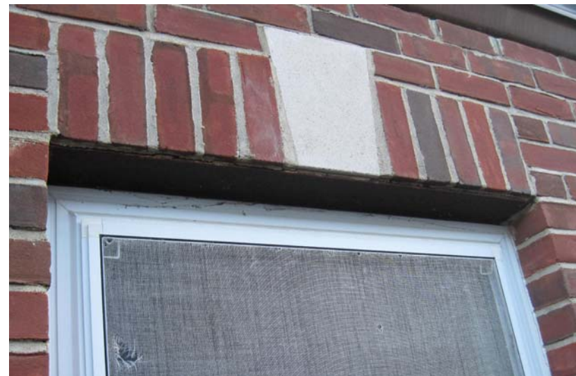
The aging corroding lintels at the five extension windows are in need of near-term replacement to avoid rust-jacking damage to the surround brick.
