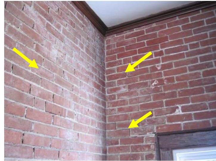
View of step-cracking and visible mortar loss noted within the egress stairwell exterior walls.
