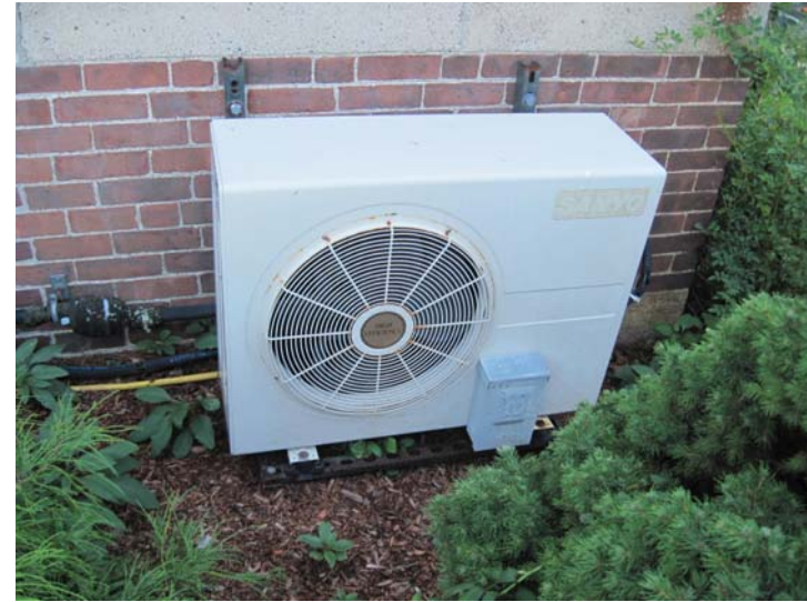
A 1.5-ton Sanyo mini-split A/C unit cools the first floor Town Clerk/Registrars Office.
