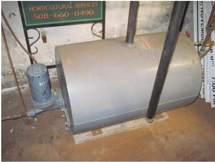
A 50-gallon boiler feed tank is assumed to date to the boiler installation; however the 1/3-hp return pump was recently installed in 2014.
