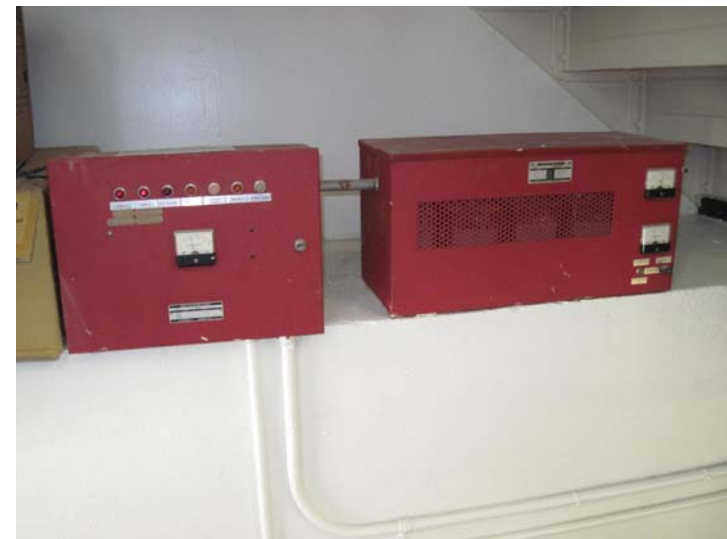
The aging zone-type fire alarm control box and outdated peripherals have far surpassed their expected useful service lives. All are in need of near term replacement.
