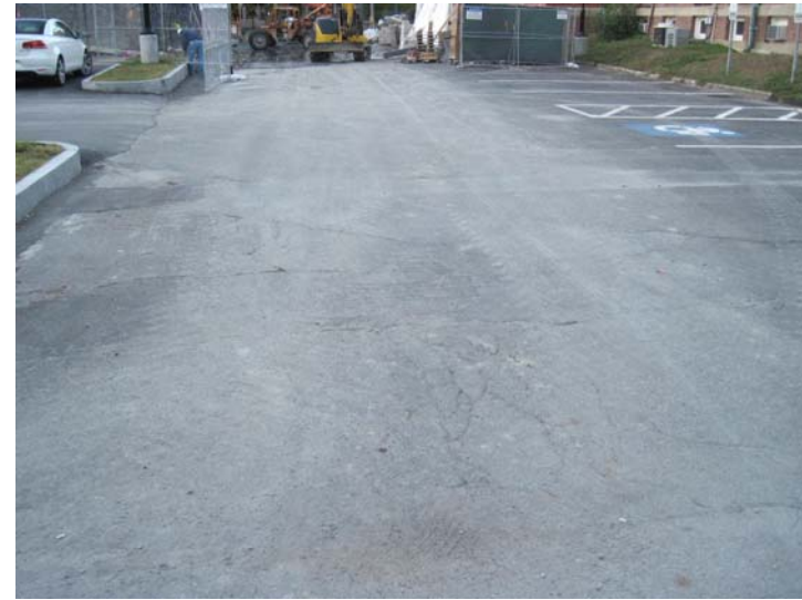
View of the rear parking lot asphalt surface conditions. Also to be resurfaced in 2016.
