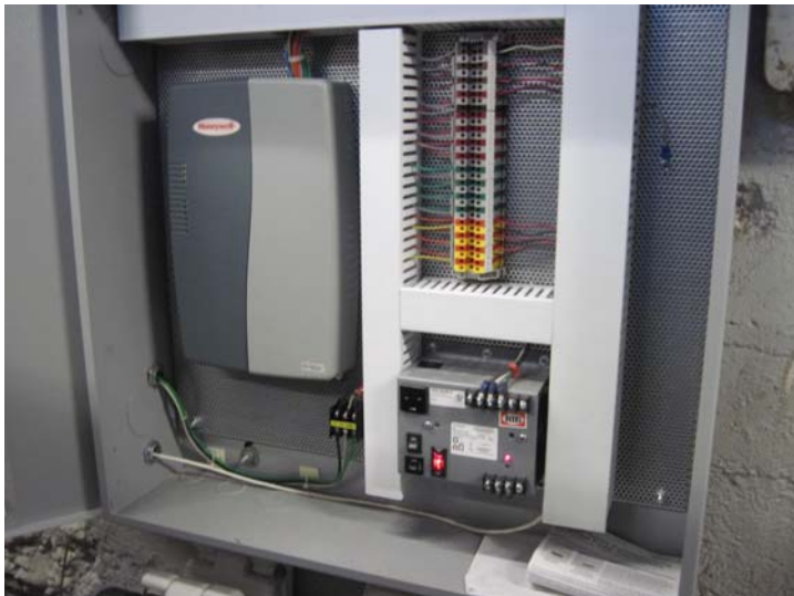
A Honeywell building automation and control network (BACnet) energy management system monitors building-wide mechanical systems performance, issues operating alerts, and provides remote troubleshooting capabilities. Westwood Town Hall • Capital Needs Assessment • © On-Site Insight
