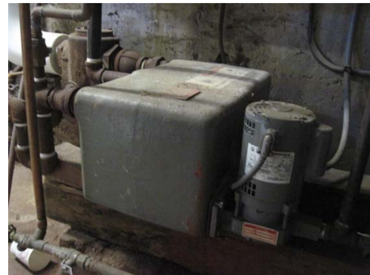
A Hoffman-Watchman 14-gallon cast-iron condensate receiver with 1/3-hp pump was installed in 2008.
