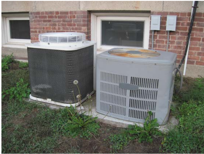
A Sanyo 2-ton ductless A/C condensing unit (left) cools the first floor general offices area; and an Allegiance-10 2-ton ducted A/C condensing unit (right) cools the second floor Selectmen Meeting Room. (Both were installed in 1995)
