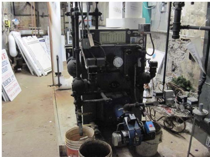
Building steam heat is provided by a 639-MBH Weil-McLain Model 80 natural gas fired steam boiler. (Installed approximately 2000)
