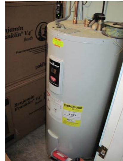
Building domestic hot water is produced by a Bradford-White 40-gallon electric hot water tank.
