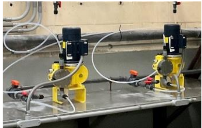
New Chemical Feed Pumps
