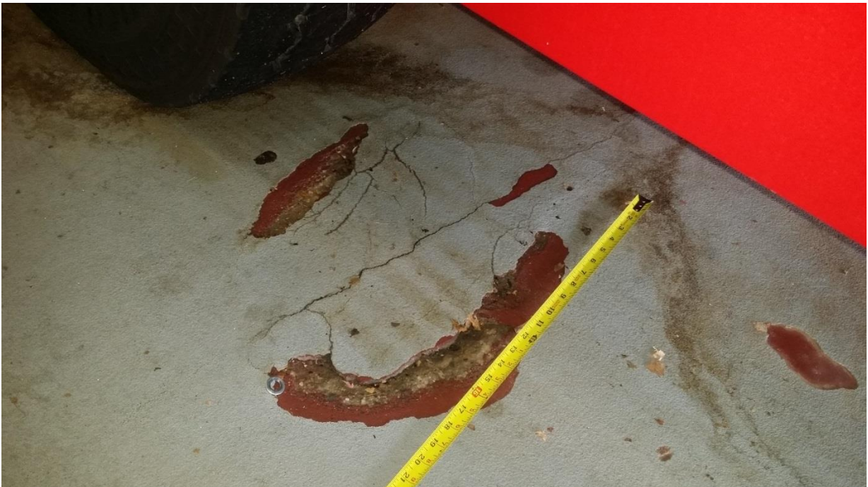
Photo 4 – Large spall where epoxy coating is damaged on the topside of the elevated slab.
