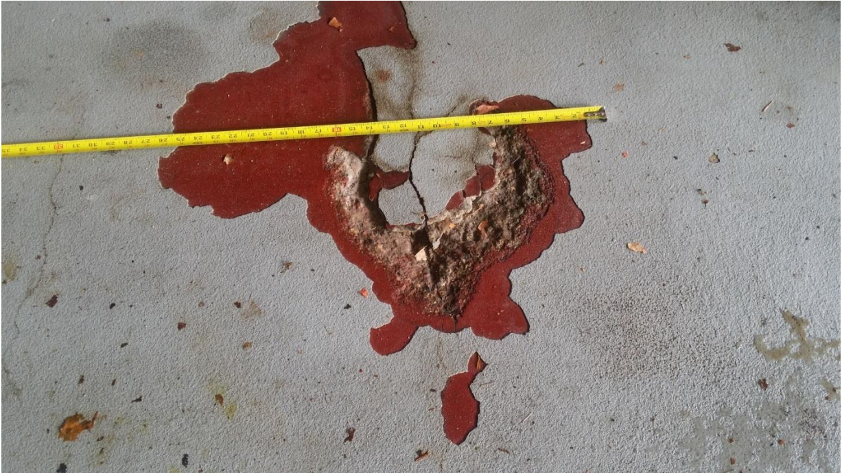
Photo 5 – Large spall where epoxy coating is damaged on the topside of the elevated slab.
