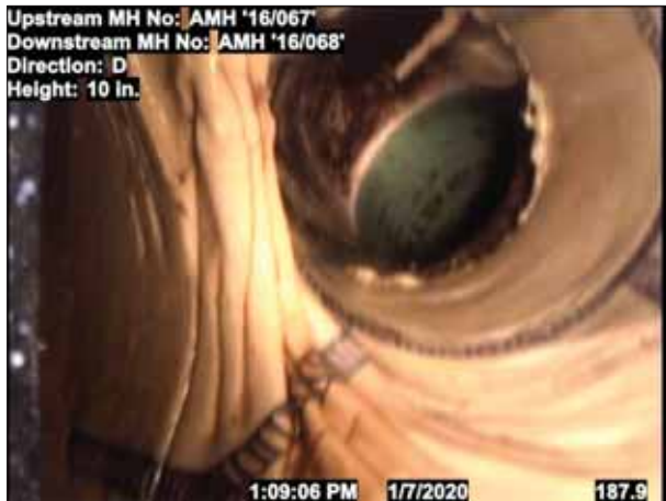
Photo: 1_1_5_24012020_080534_B.jpg, VCR No.: 123 189FT, Tap Factory Made, at 10 o'clock, 6", within 8 inches of joint: NO
