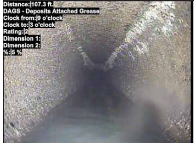
Photo: 14_013-14_017-20181116-091123.JPG At: 107.3 ft. 9/3 DAGS - Deposits Attached Grease Joint: Yes 5 %
