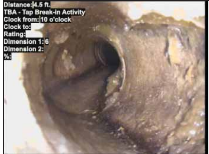
Photo: 10_078-10_079-04292020-TBA-4.5 ft.-120745.JPG At: 4.451 ft. 10/. TBA - Tap Break-in Activity Joint: No
