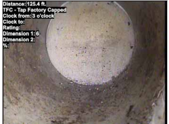
Photo: 14_070-14_071-20181116-115817.JPG At: 125.4 ft. 3/. TFC - Tap Factory Capped Joint: No
