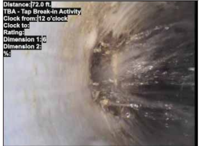
Photo: 16_067-16_068-04302020-TBA-72.0 ft.-112123.JPG At: 72.008 ft. TBA - Tap Break-in Activity Joint: No 12/.
