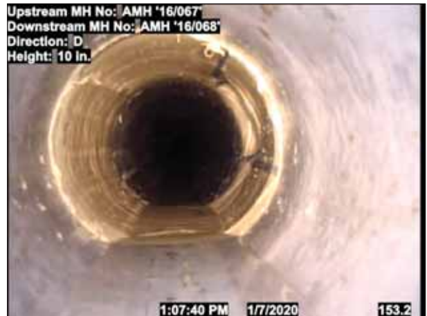
Photo: 1_1_4_24012020_080410_A.jpg, VCR No.: 123 155FT, Tap Factory Made, at 03 o'clock, 6", within 8 inches of joint: NO LAT 15-3 2' LCR INSTALLED
