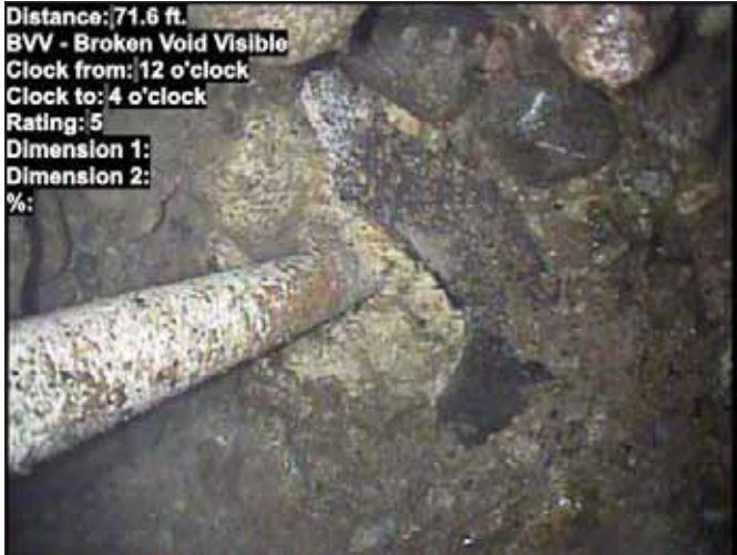
Photo: 14_071-14_013-20181116-090045.JPG At: 71.6 ft. 12/4 BVV - Broken Void Visible Joint: No
