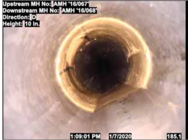
Photo: 1_1_5_24012020_080523_A.jpg, VCR No.: 123 189FT, Tap Factory Made, at 10 o'clock, 6", within 8 inches of joint: NO
