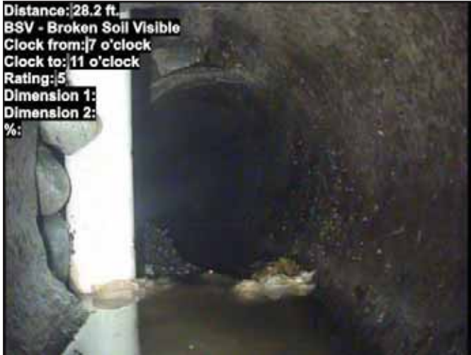
Photo: 14_071-14_013-20181116-120243.JPG At: 28.2 ft. 7/11 BSV - Broken Soil Visible Joint: No
