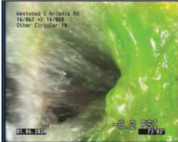
Photo: 3_3_2_06012020_153433_A.JPG, 00:00:00 Lateral Tested Failed Grouted (GAL), Retested Passed
