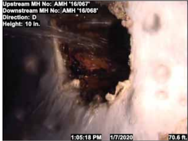
Photo: 1_1_2_24012020_080123_A.jpg, VCR No.: 123 72FT, Tap Factory Made, at 12 o'clock, 6", within 8 inches of joint: NO-GROUT ONLY
