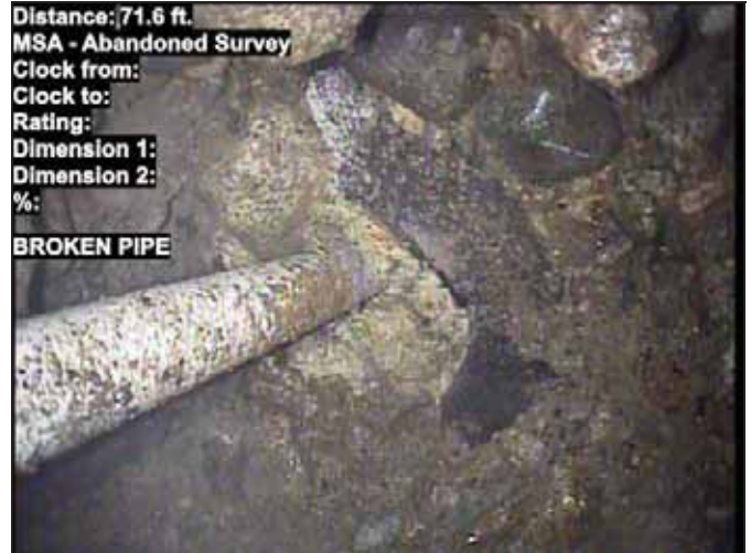
Photo: 14_071-14_013-20181116-090119.JPG At: 71.6 ft. MSA - Abandoned Survey Joint: No BROKEN PIPE
