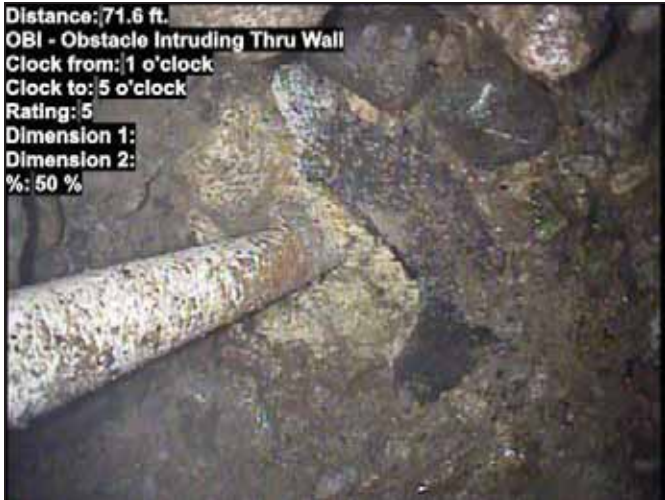
Photo: 14_071-14_013-20181116-090054.JPG At: 71.6 ft. 1/5 OBI - Obstacle Intruding Thru Wall Joint: No 50 %
