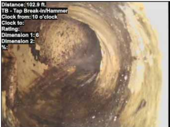
Photo: 16_067-16_068-04302020-TB-102.9 ft.-112235.JPG At: 102.868 ft. TB - Tap Break-in/Hammer Joint: No 10/.
