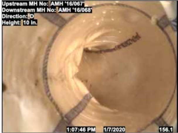
Photo: 1_1_4_24012020_080422_B.jpg, VCR No.: 123 155FT, Tap Factory Made, at 03 o'clock, 6", within 8 inches of joint: NO LAT 15-3 2' LCR INSTALLED
