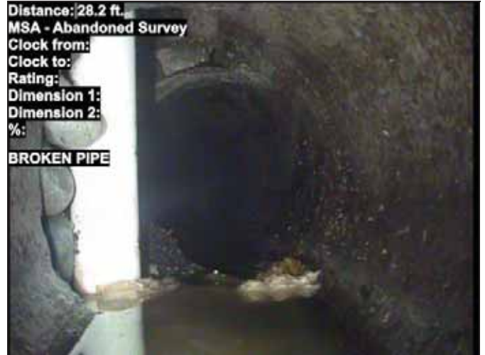
Photo: 14_071-14_013-20181116-120319.JPG At: 28.2 ft. MSA - Abandoned Survey Joint: No BROKEN PIPE
