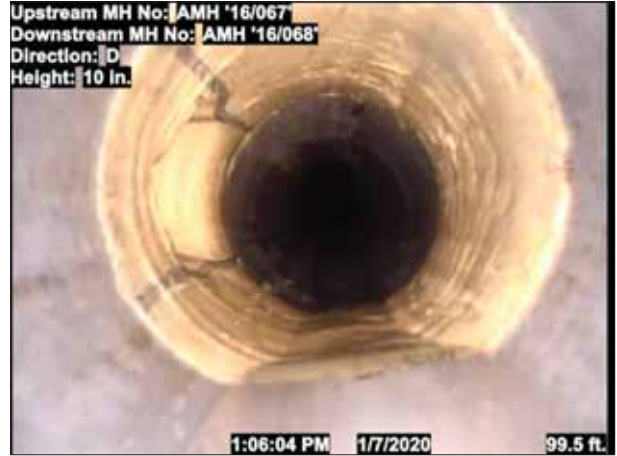
Photo: 1_1_3_24012020_080248_A.jpg, VCR No.: 123 102FT, Tap Factory Made, at 09 o'clock, 6", within 8 inches of joint: NO-LAT 15-2 2' LCR INSTALLED
