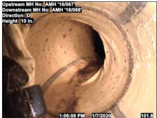
Photo: 1_1_3_24012020_080259_B.jpg, VCR No.: 123 102FT, Tap Factory Made, at 09 o'clock, 6", within 8 inches of joint: NO-LAT 15-2 2' LCR INSTALLED
