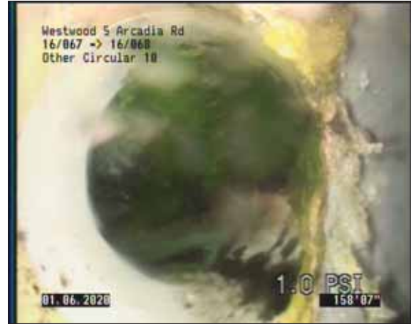
Photo: 3_3_3_06012020_160128_A.JPG, 00:00:00 Lateral Tested Failed Grouted (GAL), Retested Passed
