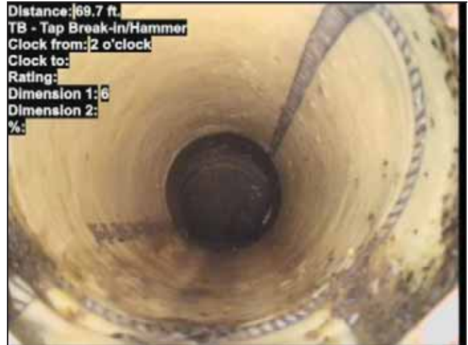
Photo: 10_078-10_079-04292020-TB-69.7 ft.-121327.JPG At: 69.733 ft. 2/. TB - Tap Break-in/Hammer Joint: No
