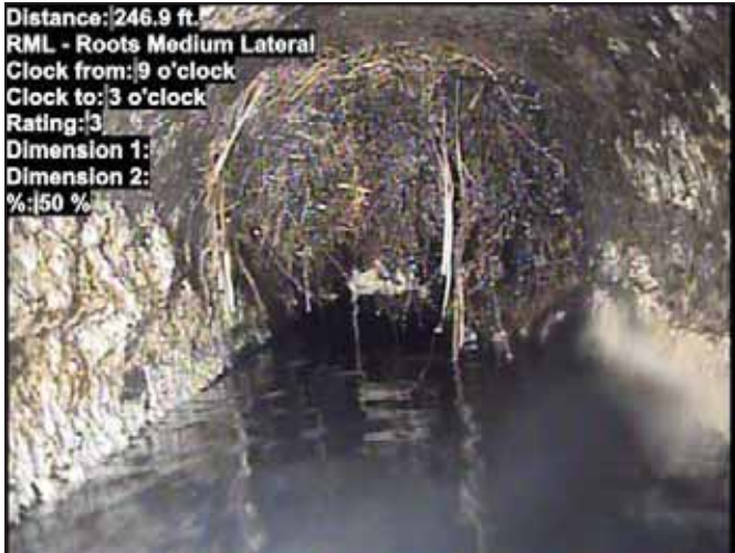
Photo: 14_013-14_017-20181116-091541.JPG At: 246.9 ft. 9/3 RML - Roots Medium Lateral Joint: No 50 %
