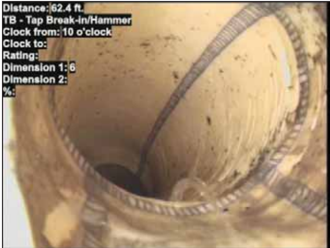
Photo: 10_078-10_079-04292020-TB-62.4 ft.-120950.JPG At: 62.413 ft. TB - Tap Break-in/Hammer 10/. Joint: No
