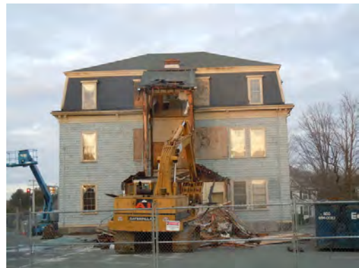
Moving the Colburn School in preparation for the construction of the New Library.
