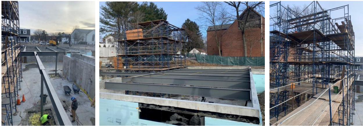
Photos showing steel framing and staging for elevator shaft at the New Wentworth Hall
