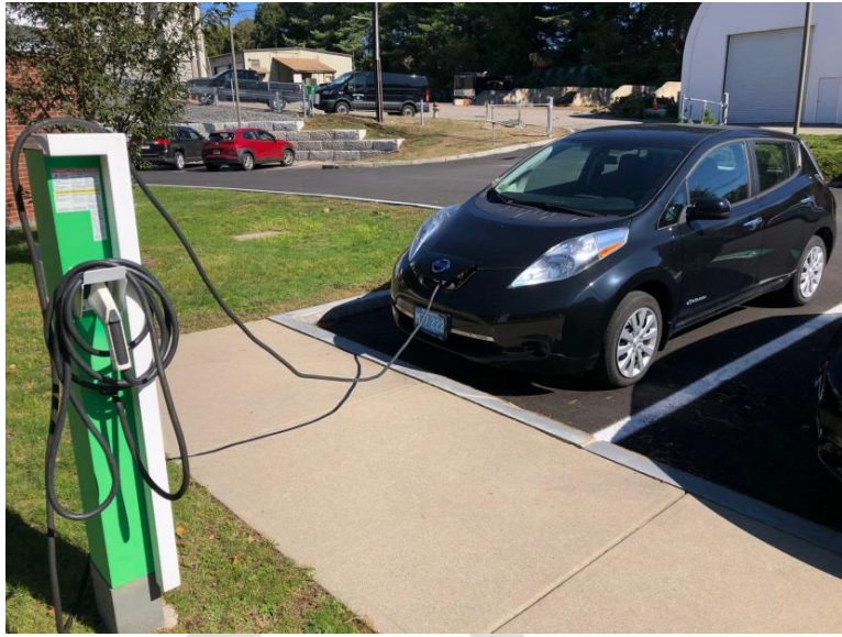
Electric Car Station at Carby Municipal Offices
