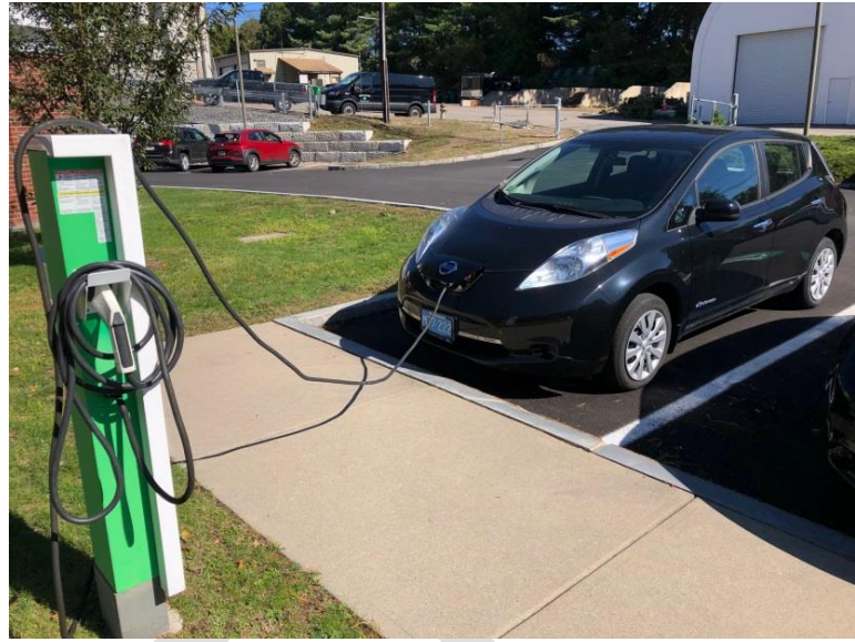
Electric Car Station at Carby Municipal Offices
