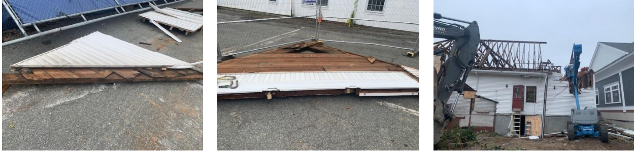
Photos showing removal of wall panels from Old Wentworth Hall for incorporation in New Wentworth Hall
