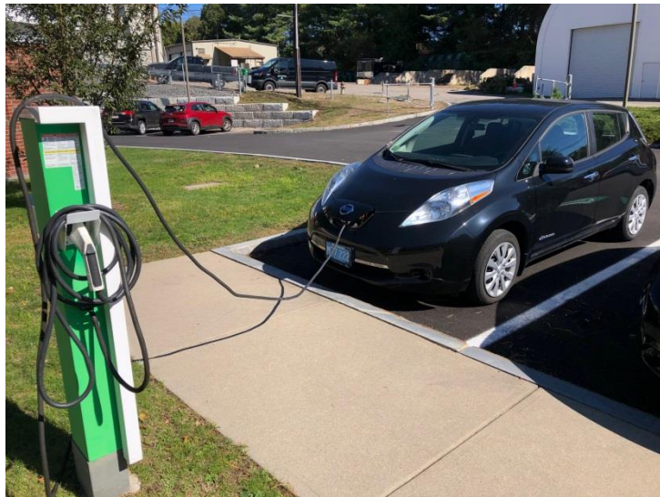
Electric Car Station at Carby Municipal Offices
