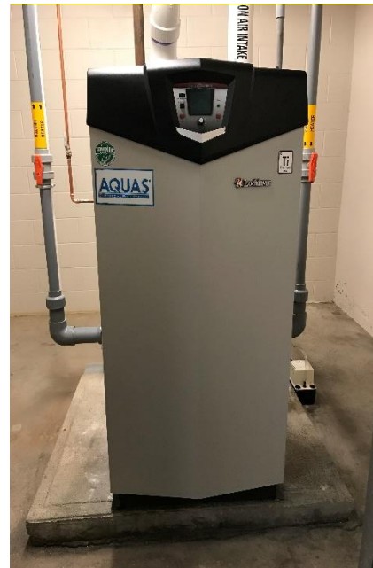
State of the art Pool Boiler
