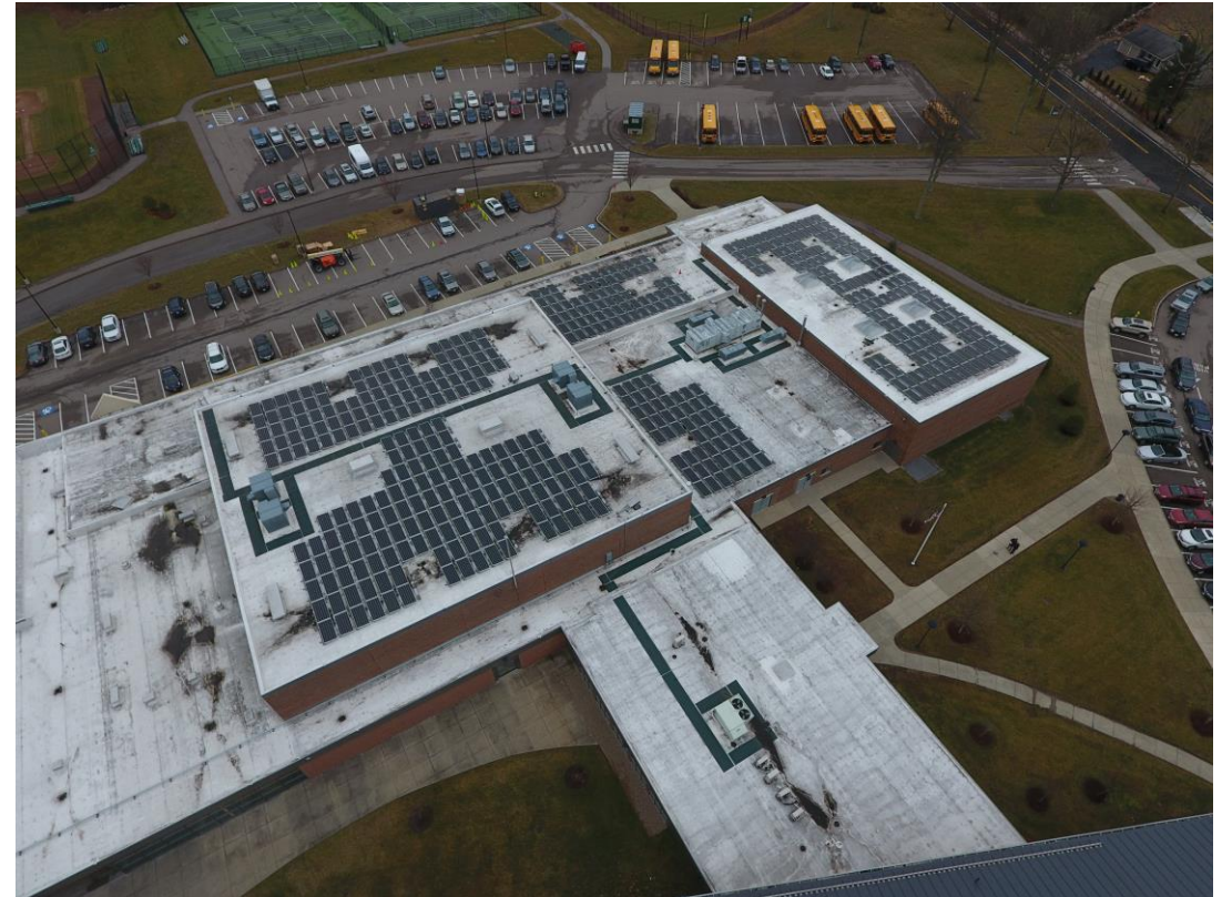
Westwood High School – Rooftop Solar PV Array (Phase I)
