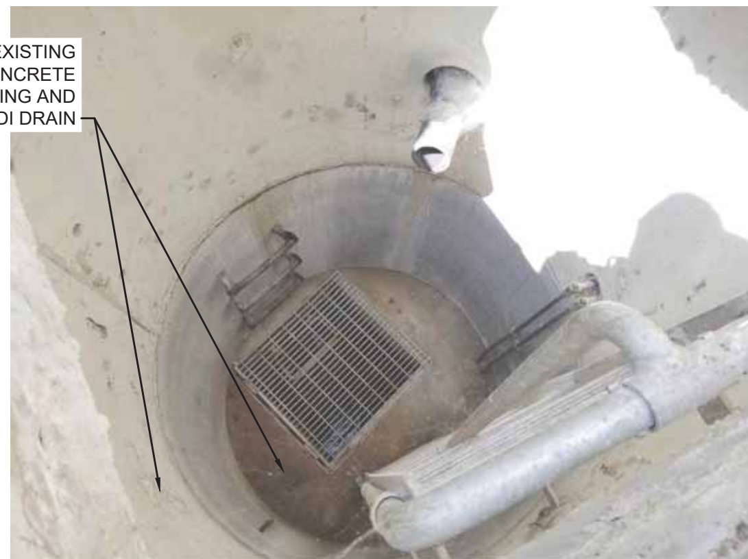
P2: WET WELL LANDING
