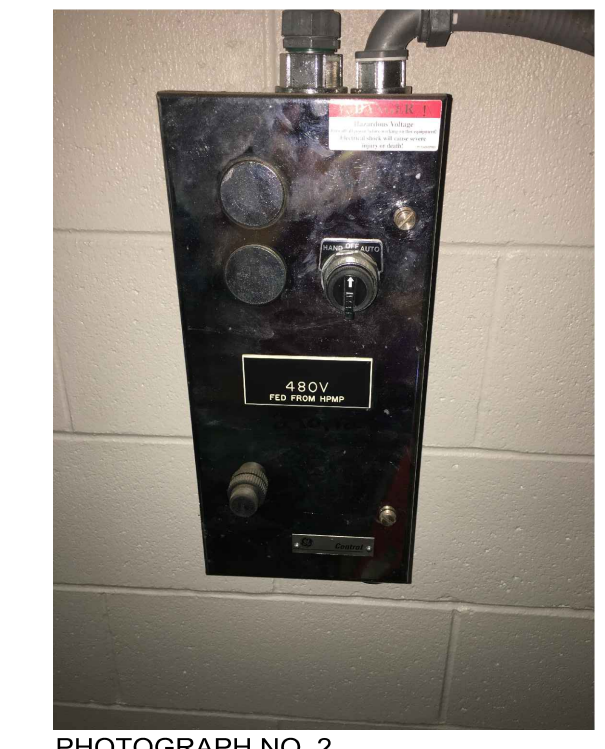
PHOTOGRAPH NO. 2 EXISTING HAND-OFF-AUTO SWITCH FOR THE EXISTING POOL CIRCULATING PUMP TO REMAIN AND BE REUSED. PROVIDE NEW LOCKABLE DISCONNECT ON THE LINE SIDE
