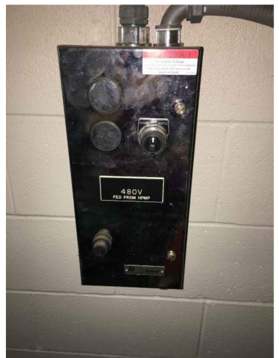
PHOTOGRAPH NO. 2 EXISTING HAND-OFF-AUTO SWITCH FOR THE EXISTING POOL CIRCULATING PUMP TO REMAIN AND BE REUSED. PROVIDE NEW LOCKABLE DISCONNECT ON THE LINE SIDE
